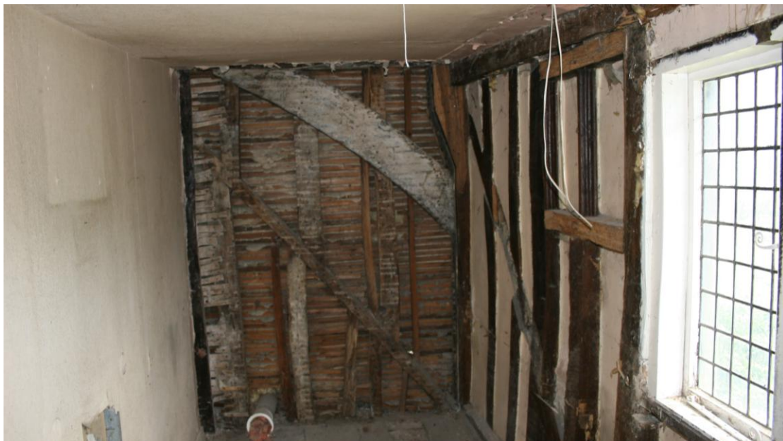
Bathroom inserted into the West Bedroom displaying curved spandrel in the studwork.
