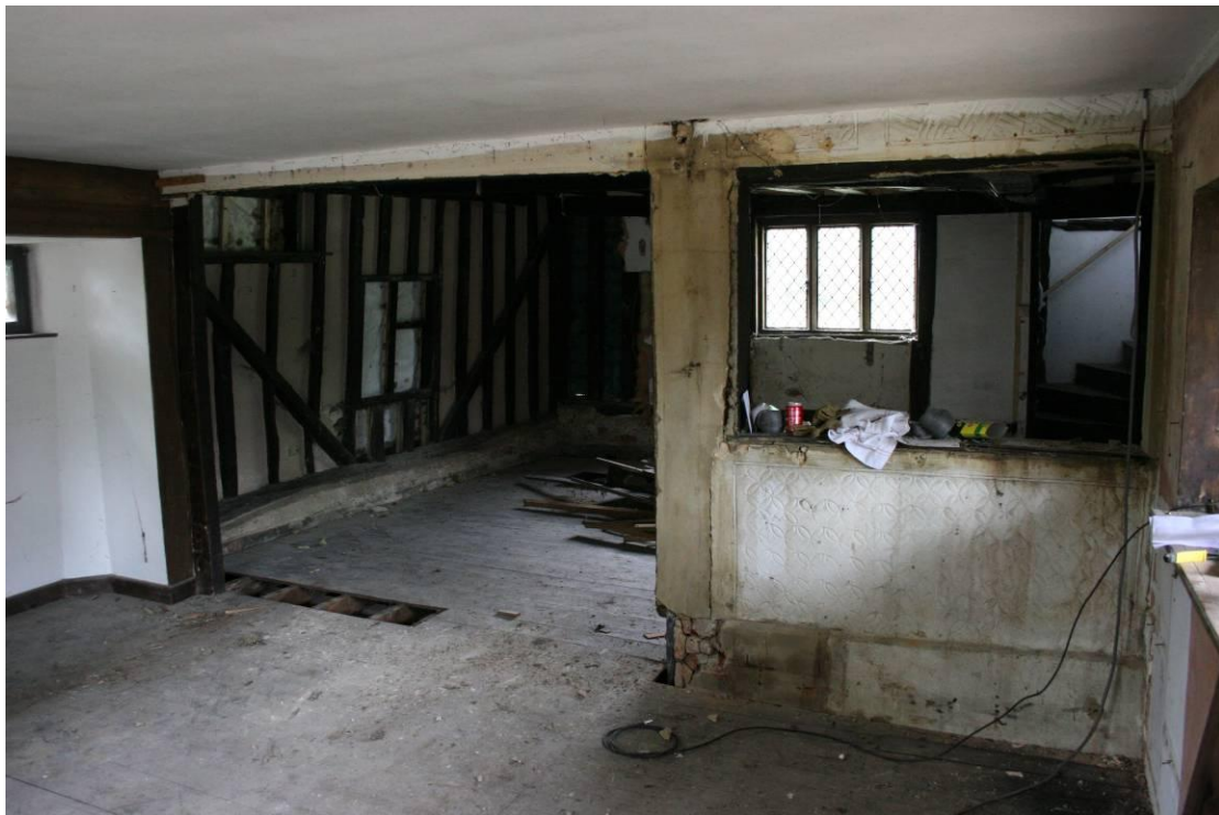
Looking NW into the Sitting Room. The former exterior wall is pargetted.
