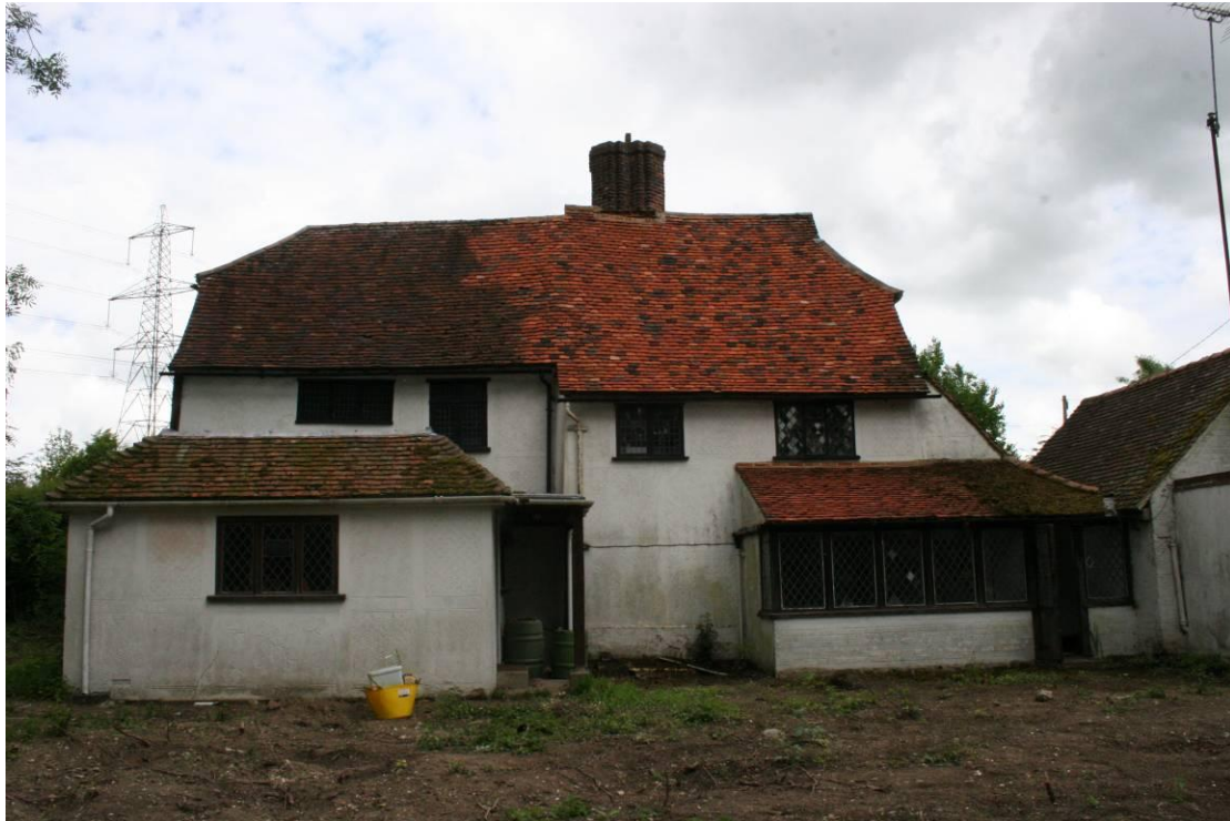
Oak Cottage. Southern Elevation. The roof is being cleaned by pressure washer.
