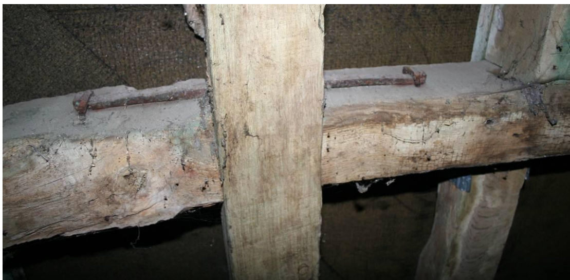
Wrought iron tie reinforcing the butt purlins as they meet at the principal rafter.
