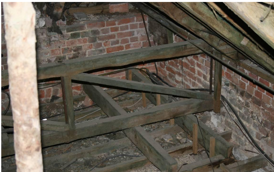
Looking SE down on the Stable ceiling at the clock platform support truss.
