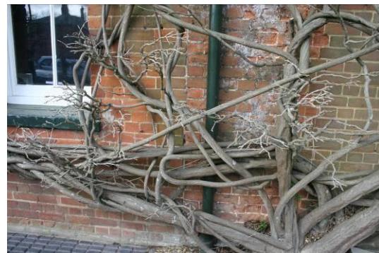
Butt joints in the brickwork by the window.
