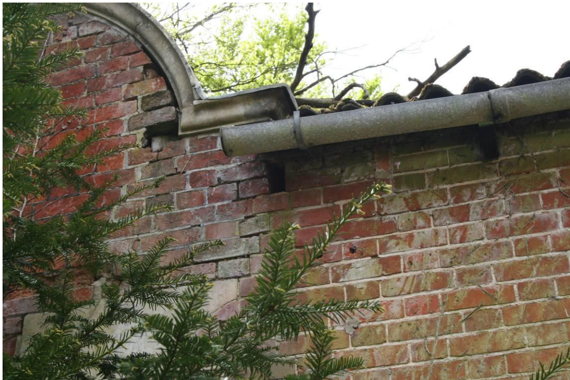
Detail of the junction of the ogee gable with the top of the Squash Court wall.
