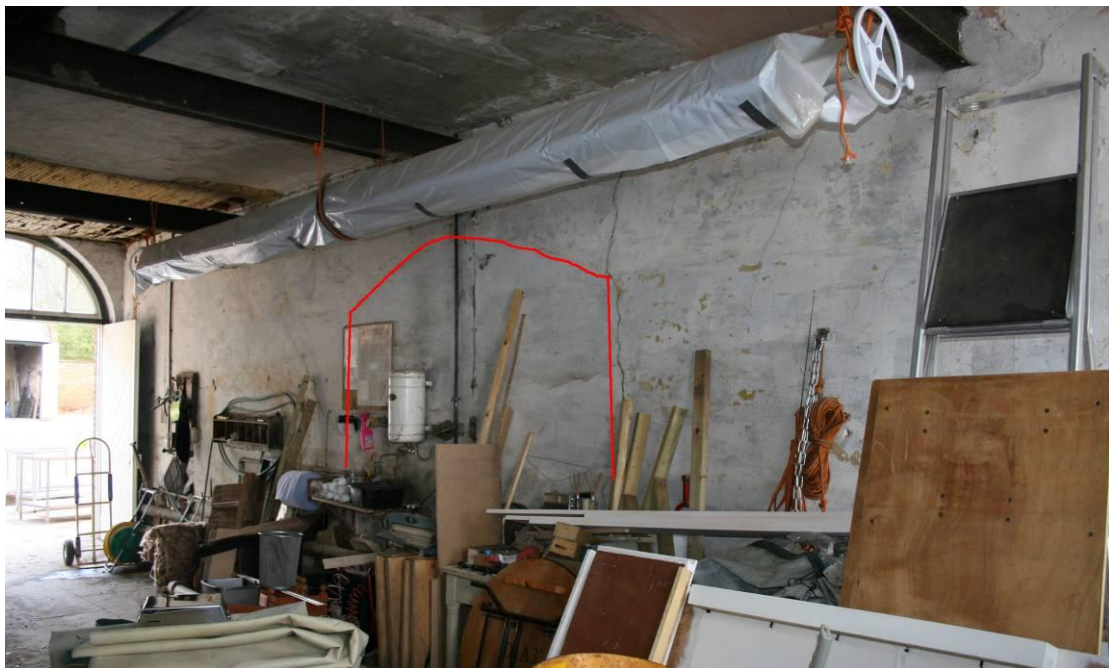
Looking SE at the south wall of the Garage. There is a blocked in archway.
