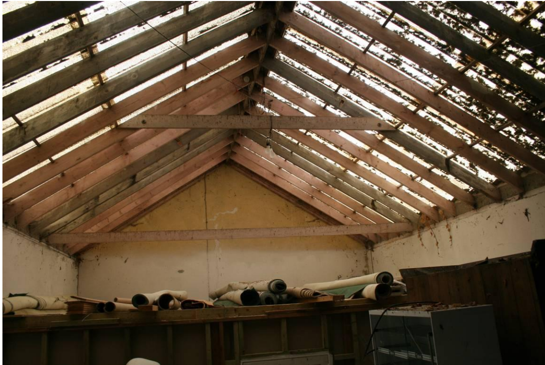
Looking NW in the Squash Court. The studwork below is the newly inserted rooms.
