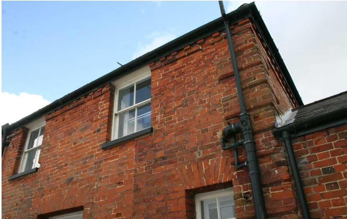
Detail of the NW elevation at the SW corner with the extension.
