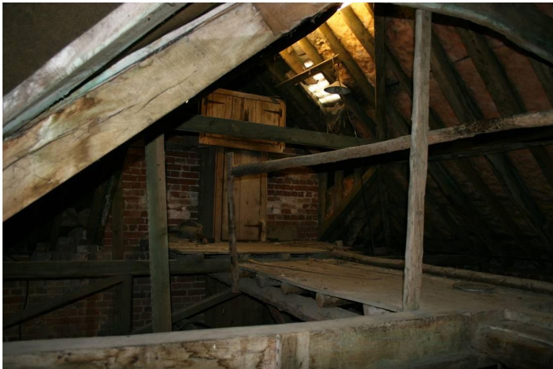
Looking SE at the clock cabinet. The rustic gantry is in poor condition.
