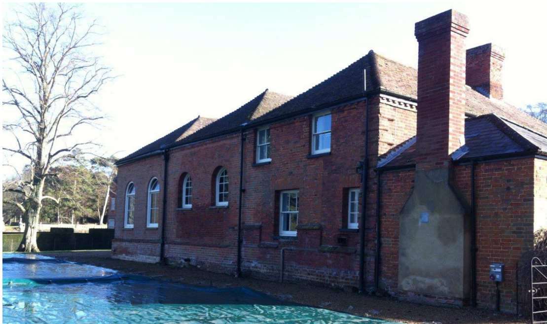
Looking NE along the length of the NW elevation. Photo by Colin Walker.
