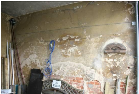
The SW wall with a fire hose reel holder.
