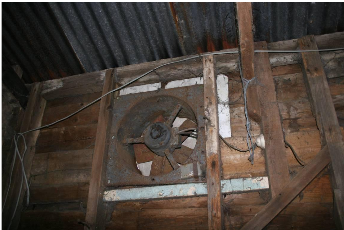
Detail of the extractor fan.
