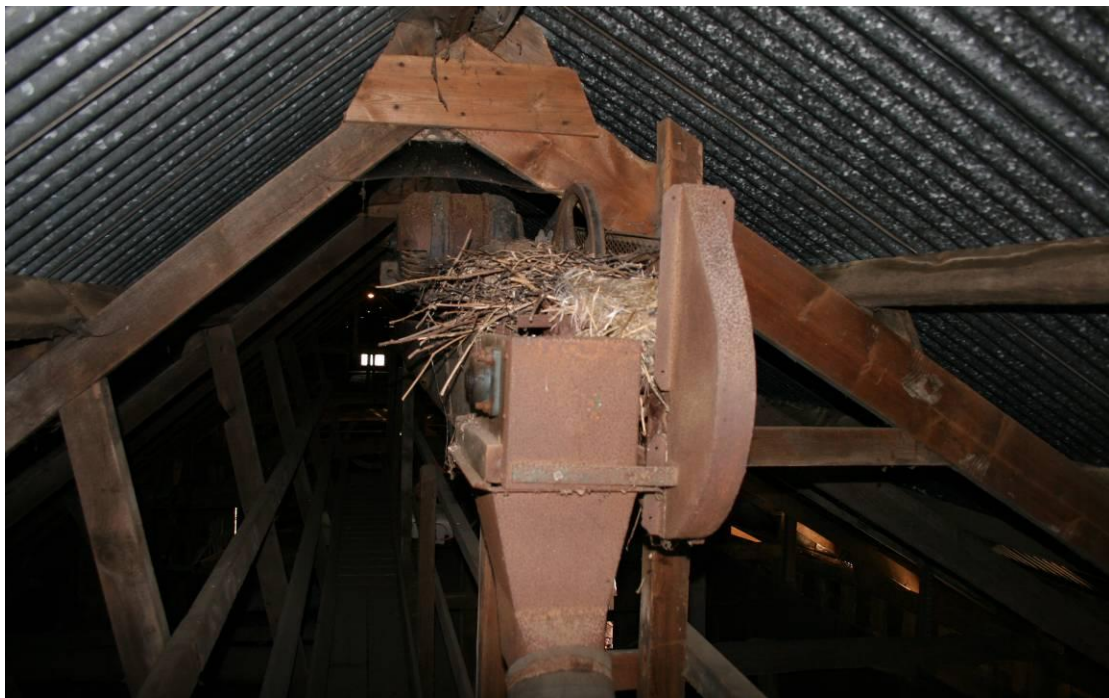
Electric motor gear to run the chain drive in the roof. Looking E from the W end.
