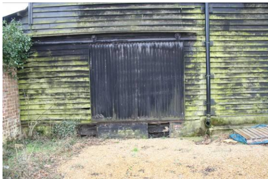
The sliding steel door to Bay 5..
