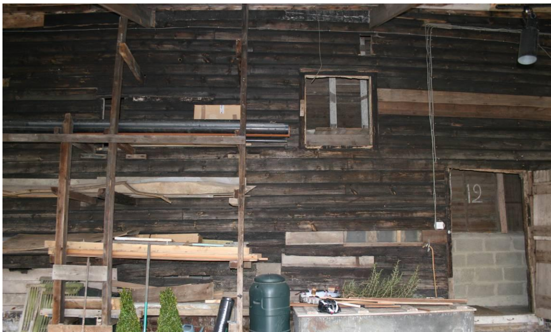
The southern elevation of Bays W2 and W3 in the West Frame.
