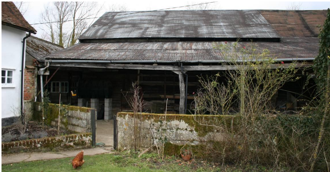
The more recent roof of the West Frame above the Open Shelter.
