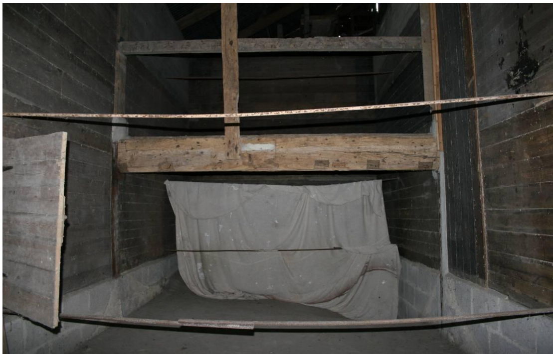
Looking W into the eastern silo. Note the main joist that originally supported a floor.
