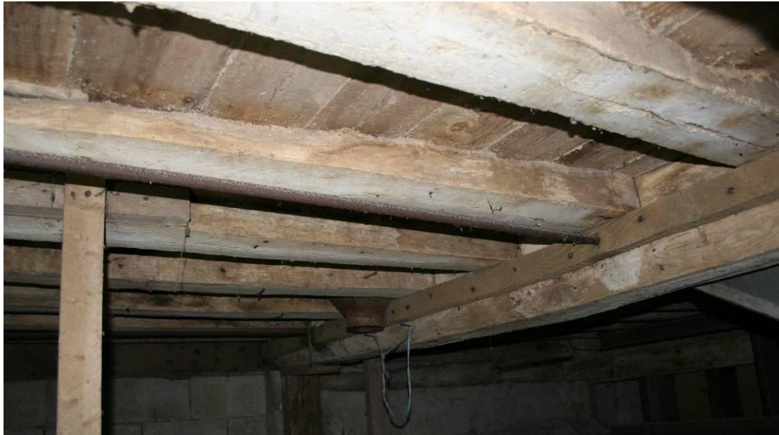
The granary floor has flat joists and wide elm and pine boards.
