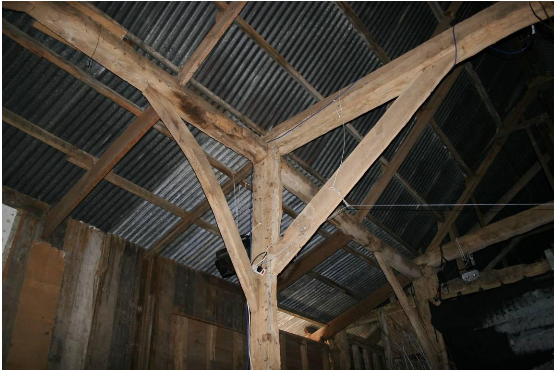
Detail of the arcade post in Truss 2, south side. Curved and straight spandrels.
