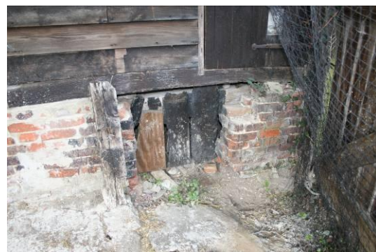
Ventilation duct for the boarded floor.
