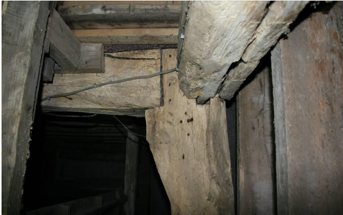
Detail of the storey post and main joist for the granary floor.
