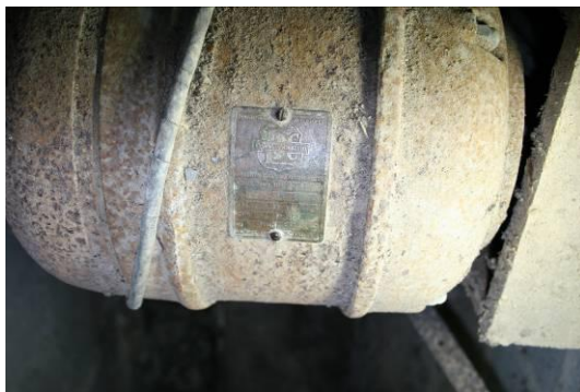
Detail of the floor motor.
