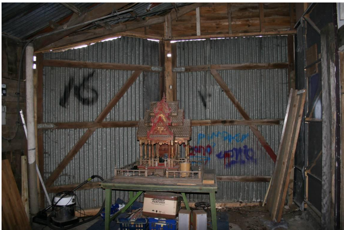
Looking E inside the Pre-dresser. The gates likely opened to admit lorries or trailers.
