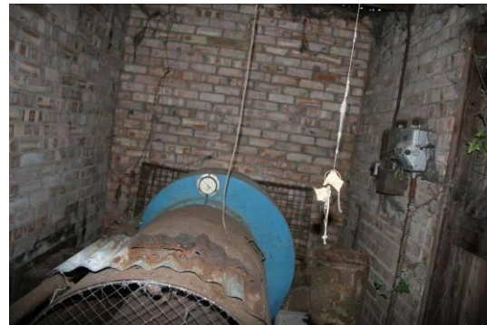
The electrically powered drier motor.
