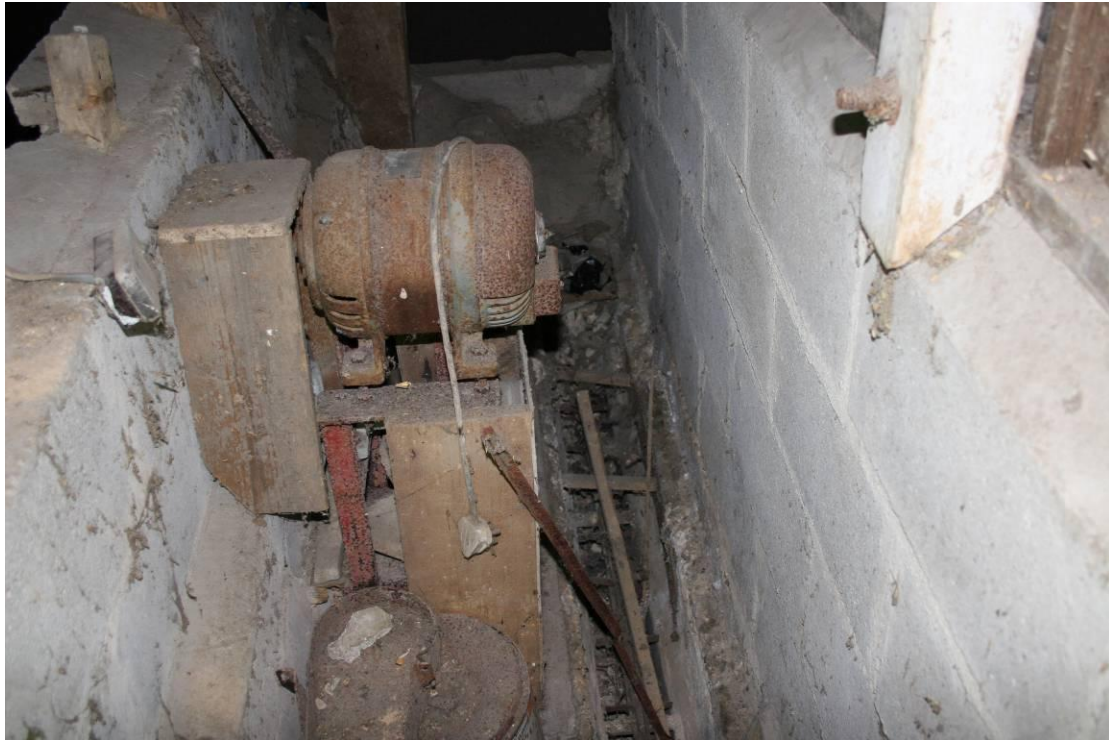
Electric motor to run the chain drive in the floor.
