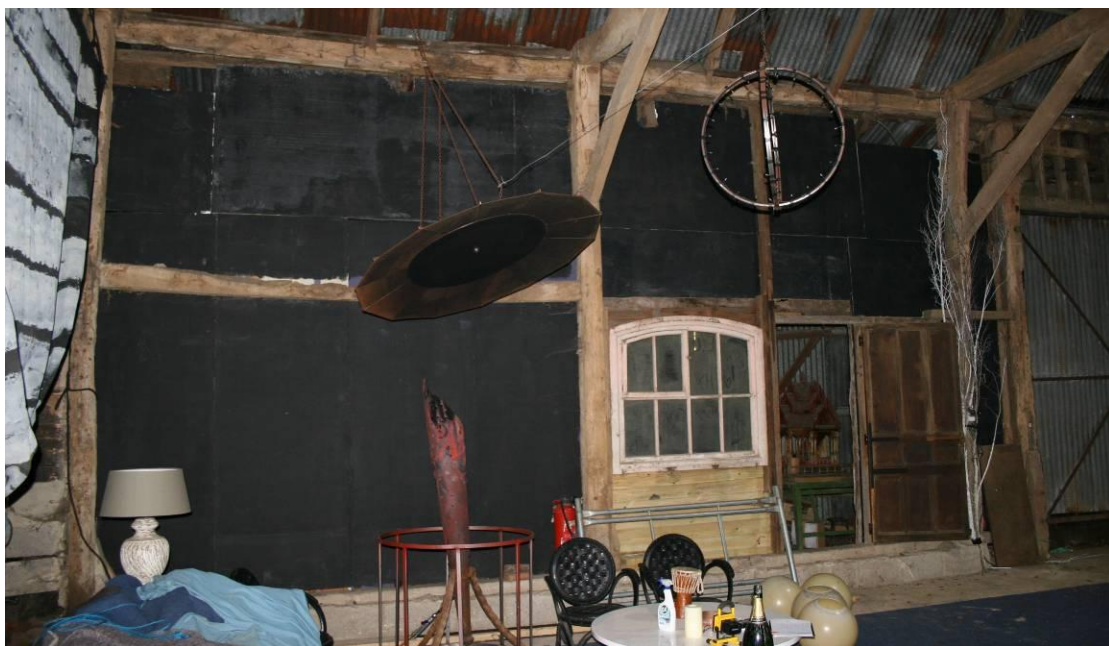
Bays 1 and 2 on the northern side. The studwork was removed for the Pre-dresser.
