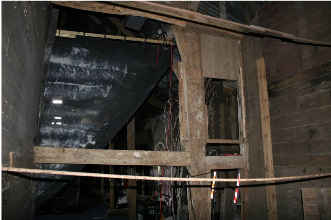
Standing in the eastern silo looking at the arcade post of the East Frame.
