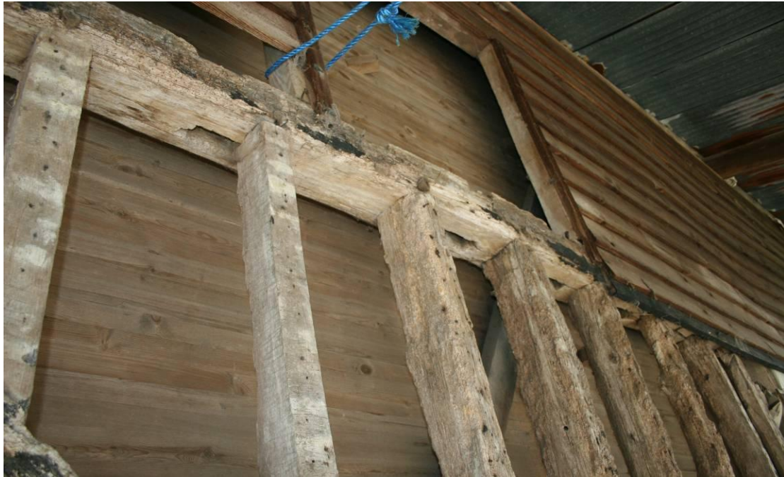
Looking up at the mid-rail in Bay E4. The shuttering is part of an old timber silo.
