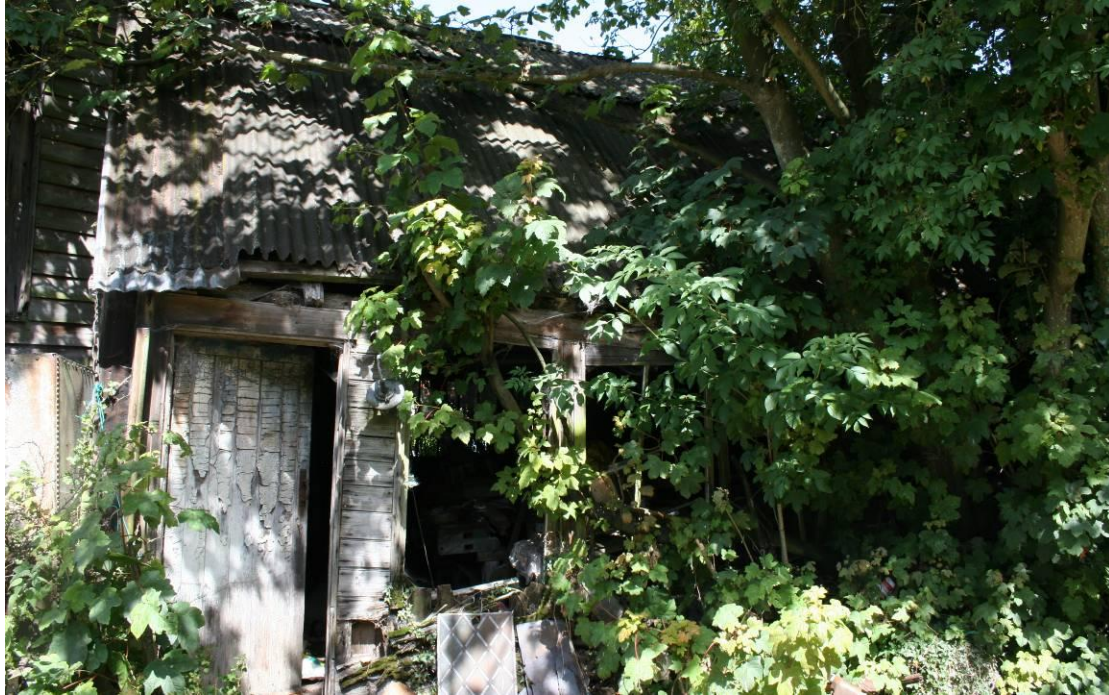
The Workshop is in parlous condition.
