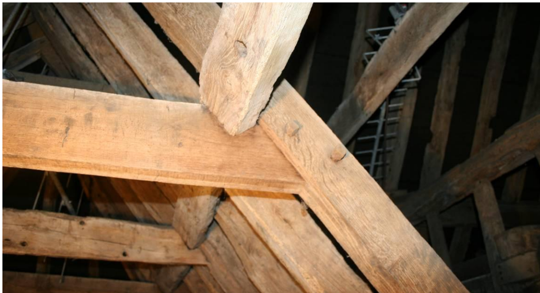
Detail of the clapsed side purlin.
