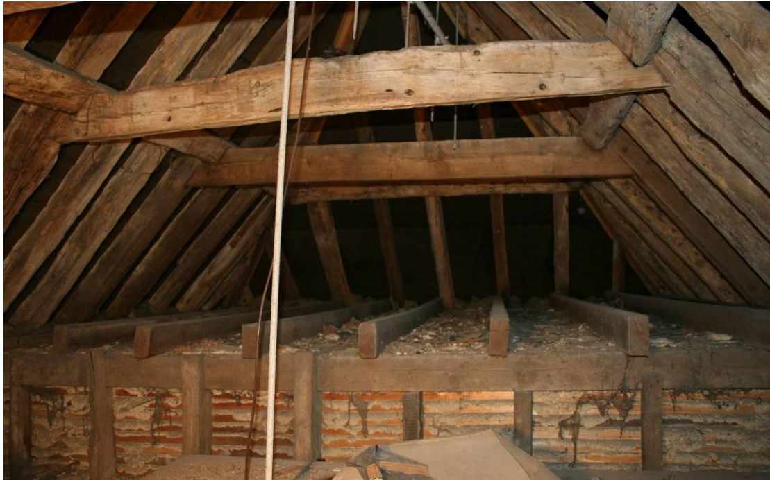
Looking S in the cross-wing roof across the ceiling of the south bedroom.
