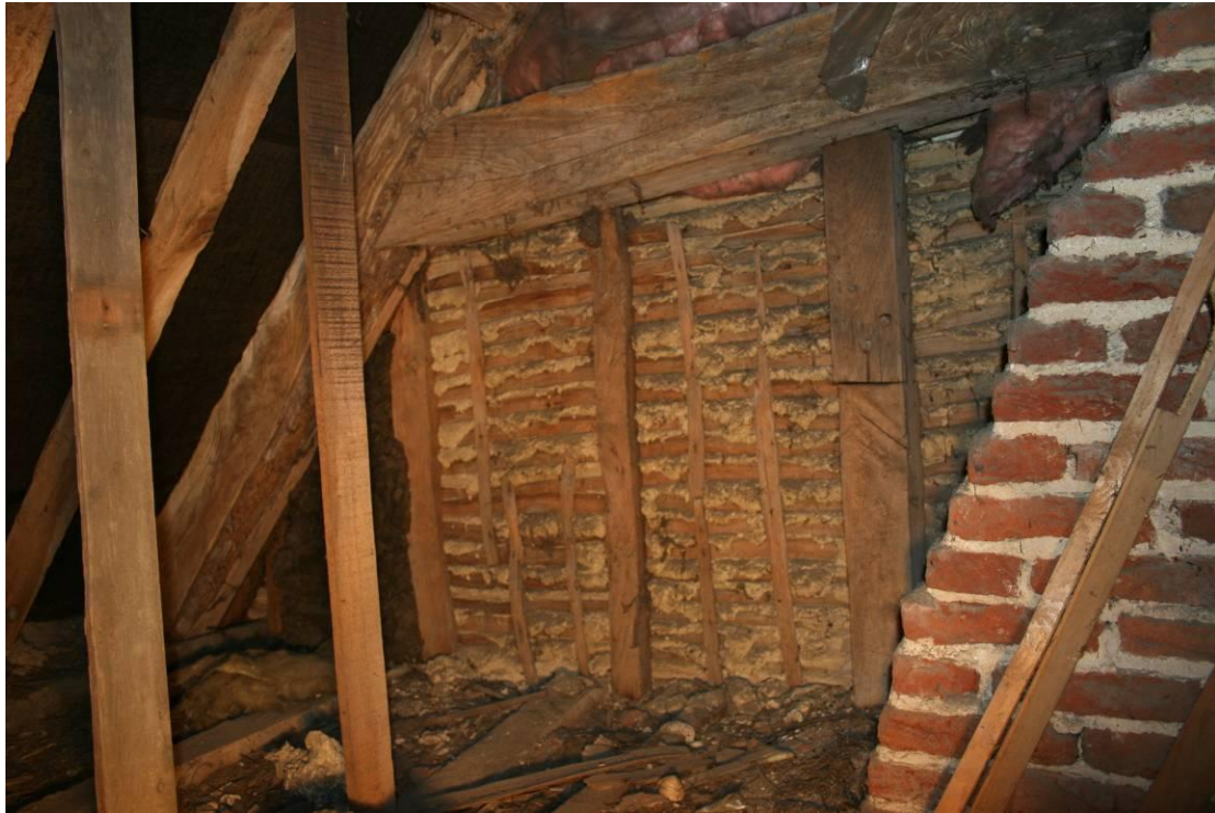
Looking SW the void above the fireplace. Note the nailed vertical laths and reused studs.
