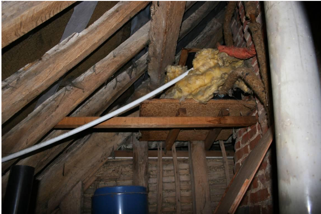
The offset butt purlin roof over the Master Bedroom in Wyndies Cottage.
