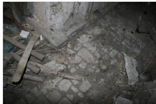
The worn floor in the Pantry.
