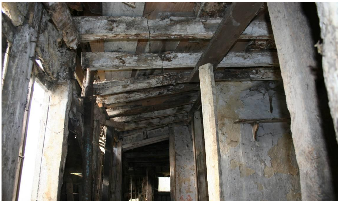
The structure of the first floor. The door frame indicates the amount of sag. Looking W.
