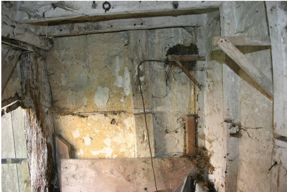
Detail of shelf supports and slot cut for other shelves. Note the tethering ring up high.
