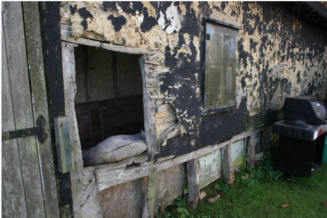
Detail of the exposed frame and lath and daub finish.
