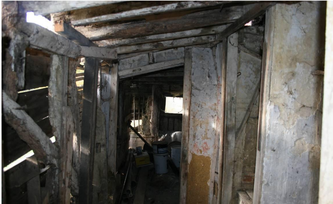
Lobby besides the firestack. Note the collapse of the frame.
