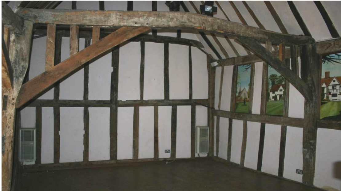
The Brew House looking N. Note the reused timbers and iron straps.
