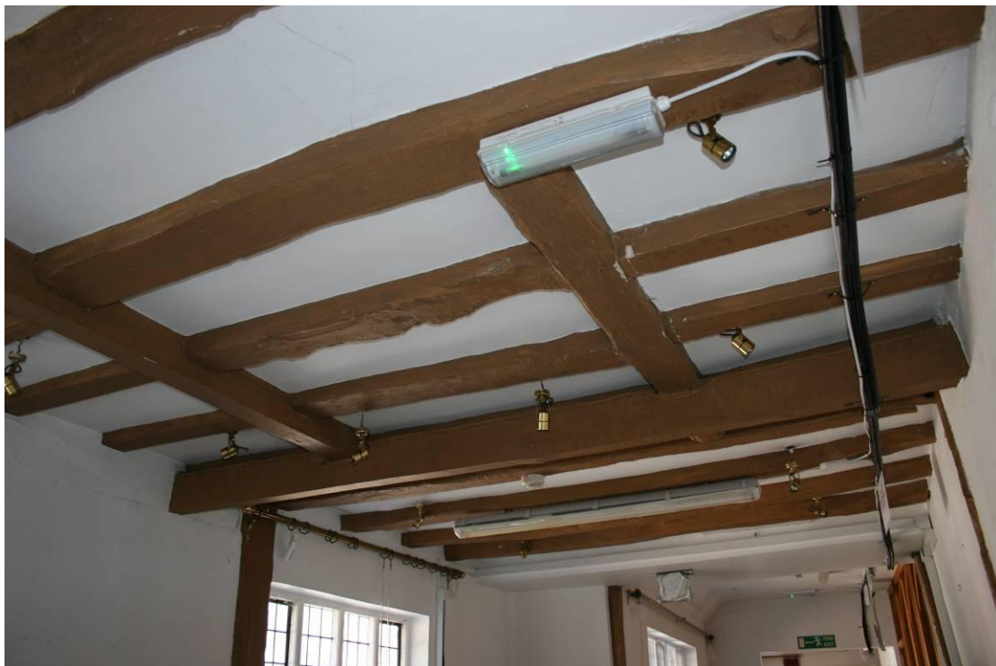
The ceiling frame of the room in the Brew House is not convincing.
