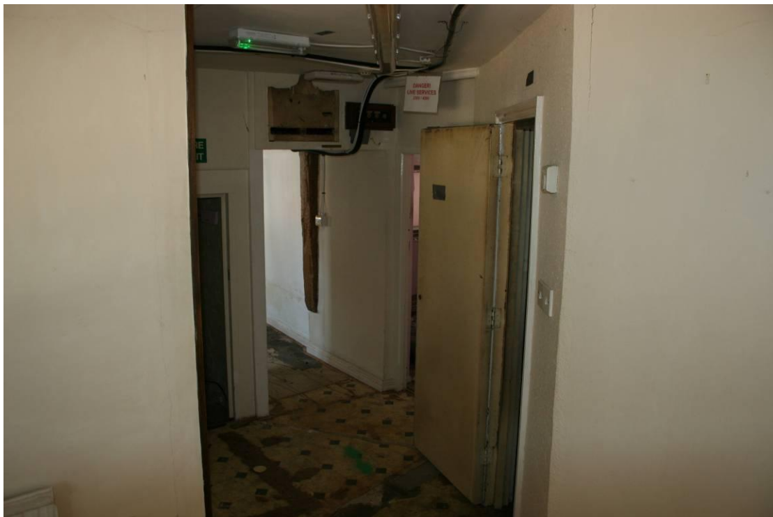
EC20th link with boiler room.
