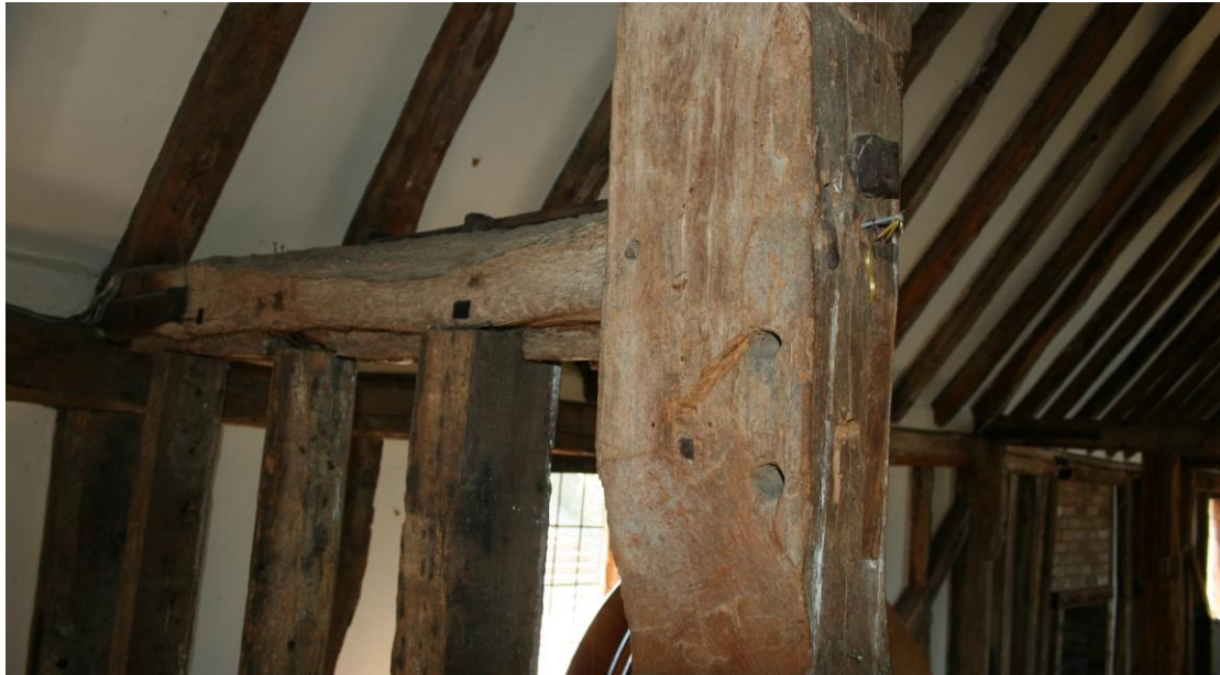
Detail of one of the arcade posts. Note the large iron nut.
