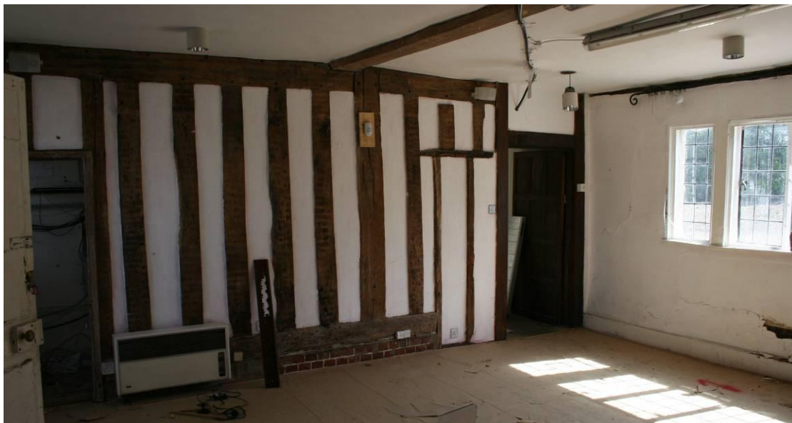
The lower wall of the cross-wing is visible in the Entrance Hall.
