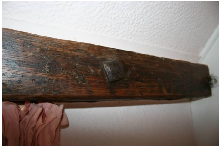
A square headed bolt in a repair clamp.
