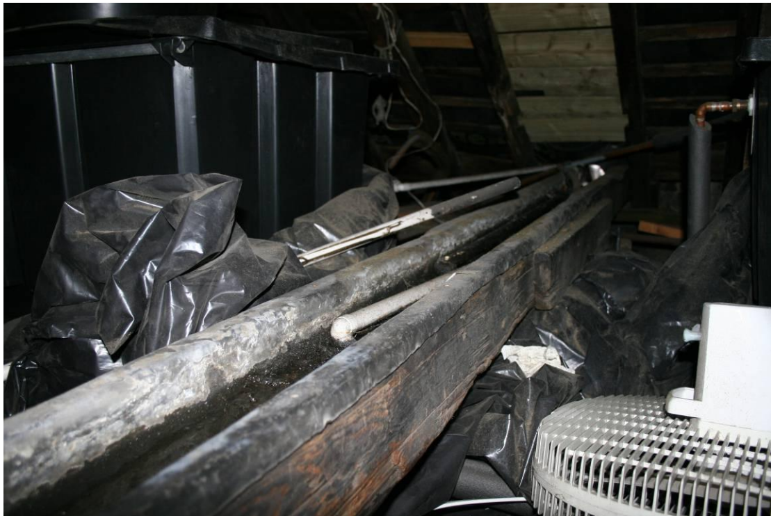
The lead lined drainage rill. Filled with moss and rubbish it needs to be cleared out soon.
