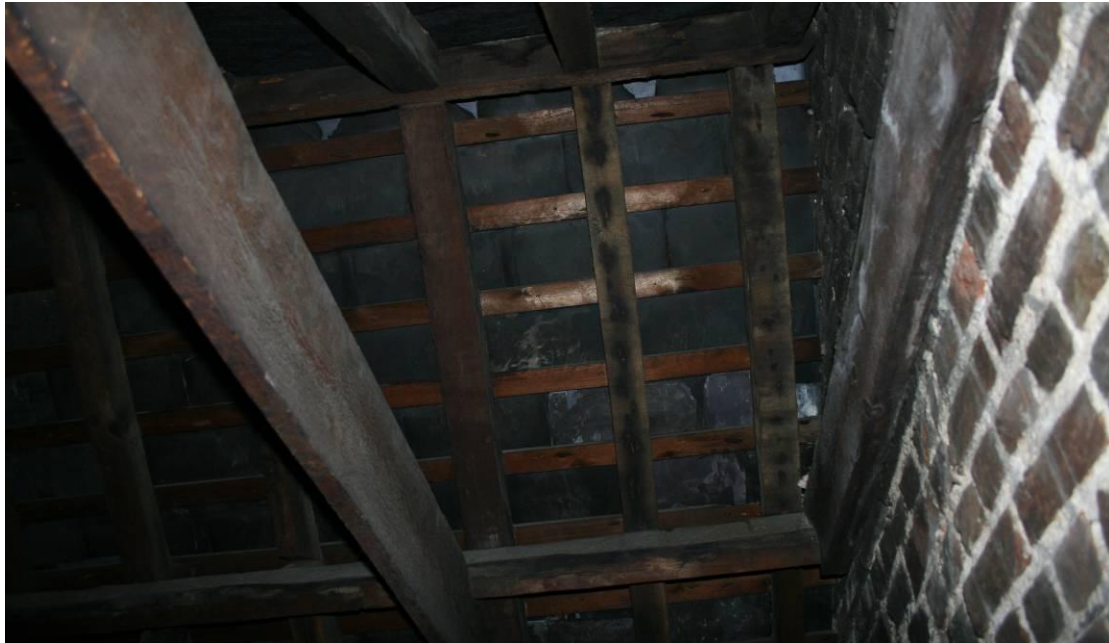
Looking upwards to the south. Note the turned over rafters and C20th machine cut battens.
