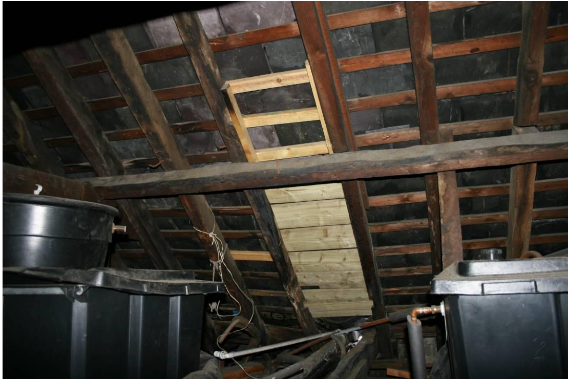
The repaired roof above the rill. Looking SW. Note also the brand named rubber membrane.
