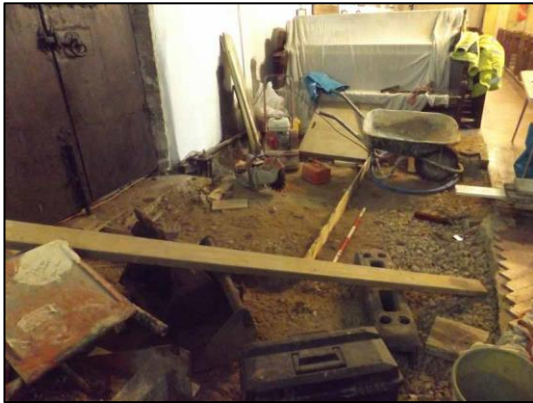
Plate 5: Ground reduction at NW corner of inside church, looking E (1m scale)
