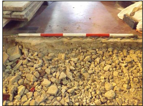
Plate 6: Ground reduction at NW corner of inside church, looking S (1m scale)
