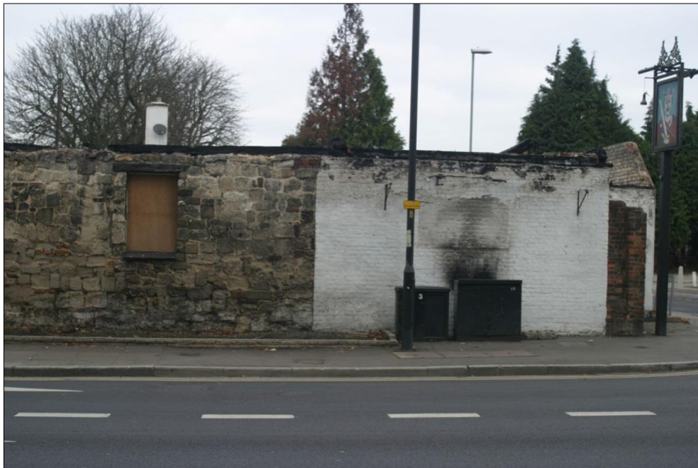
Figure 18: The eastern end of the south elevation of the Norman King after the fire (Courtesy of Will Riley)
