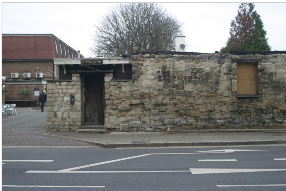
Figure 17: The south elevation of the Norman King after the fire (Courtesy of Will Riley)
