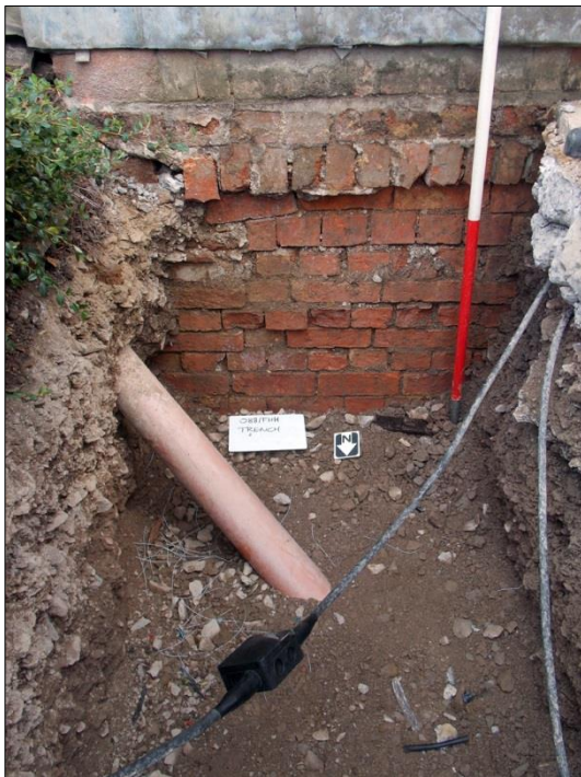
Plate 2: Northeastern end of trench and Georgian plant foundations, facing south, with 1m scale
