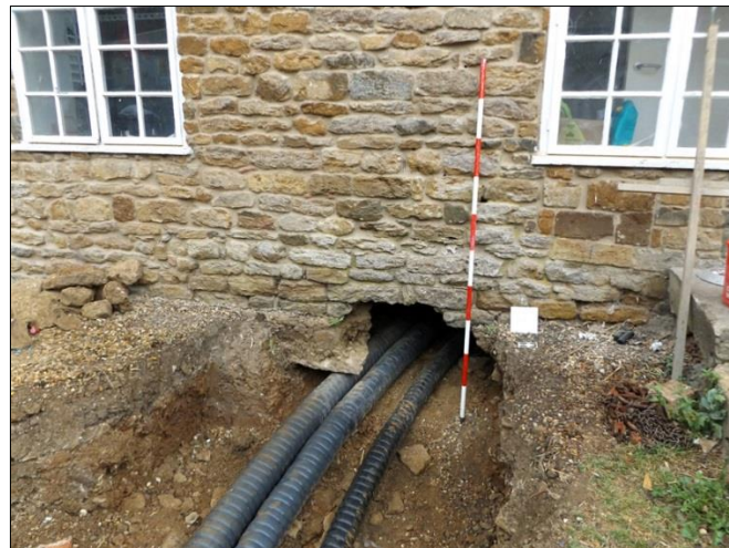
Plate 6: Southwestern end of trench with proposed plant room foundations, facing southwest, with 2m scale
