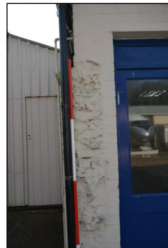
Plate 40: Shot 38. Scar of demolished wall on north elevation of the History Centre
