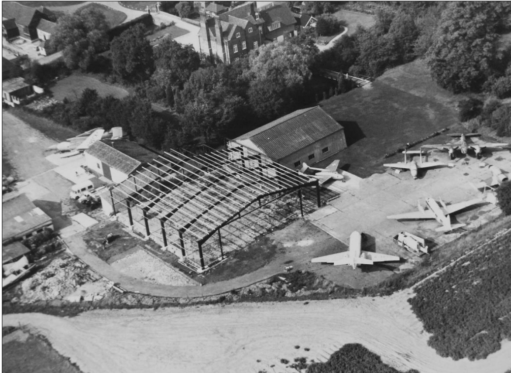
Figure 6: Aerial photograph showing the construction of a new hangar (Courtesy of the de Havilland Aircraft Heritage Centre)
