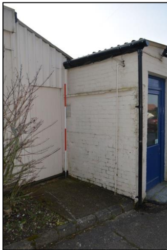
Plate 41: Shot 39. Scar of demolished wall on east elevation of the History Centre
