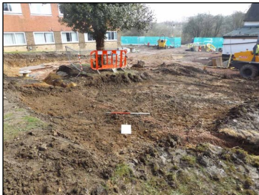
Plate 3: Strip, Map & Sample for new patio at NW corner of site, looking E (1m scale)
