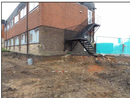
Plate 5: Strip, Map & Sample, towards the E end of site, looking N (2x1m scale)
