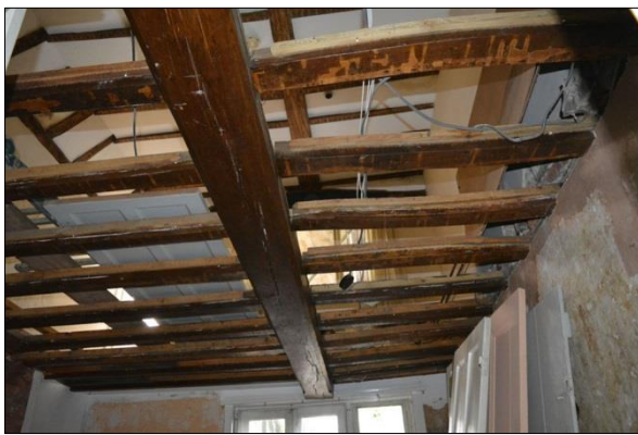
Plate 9: Fully exposed joists in Room F8 from below
