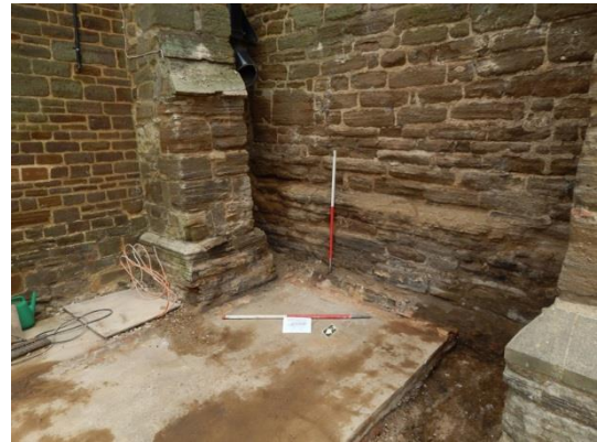
Plate 2: Shot 12. Junction between north aisle and the western tower following boiler house demolition.
