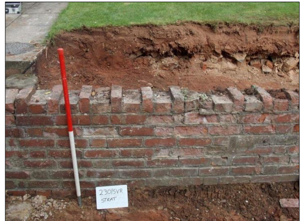
Plate 4: Retaining wall and reduced patio level from the footprint of the new extension
