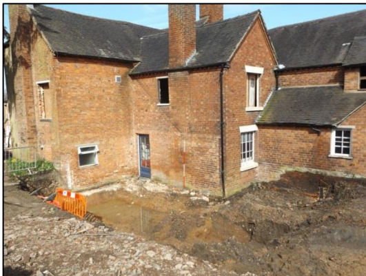
Plate 9: Trench 3, in relation to existing buildings on the site, looking NW (2m scale)
