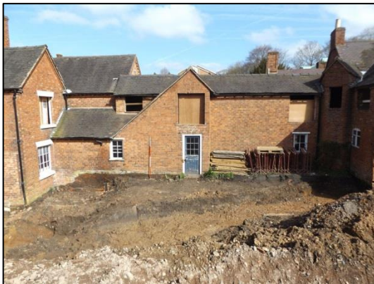
Plate 15: Trench 4, in relation to existing buildings on the site, looking NNE (2m scale)
