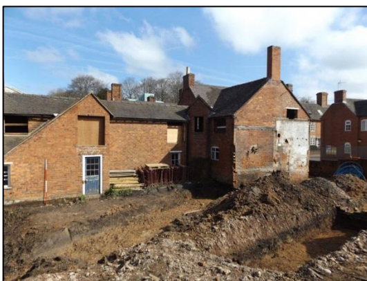
Plate 22: Trench 5 & 4, in relation to existing buildings on the site, looking NE (2m scale)
