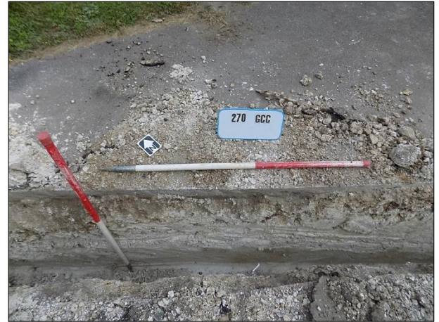
Plate 23: General stratigraphy of man-hole and service trench underlying church pathway, view NE
