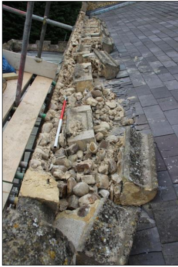
Plate 19: Watching brief, collapsed north nave parapet (48)
