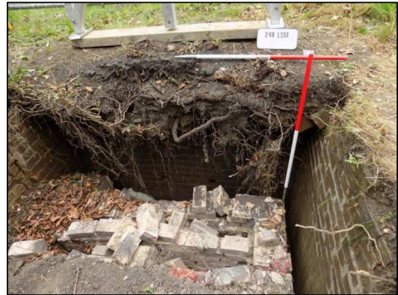
Plate 10: Rooting damage looking south
