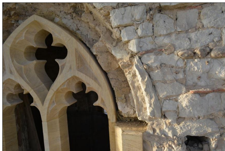
Plate 14: East window: remains of clunch hood mould and put log hole
