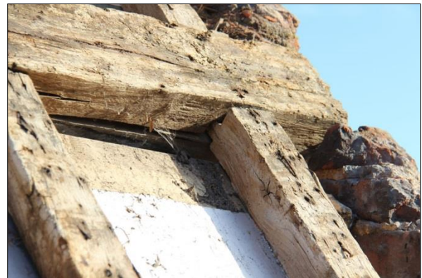
Plate 10: West range roof, west side: off-centre tenon joint between purlin and common rafter
