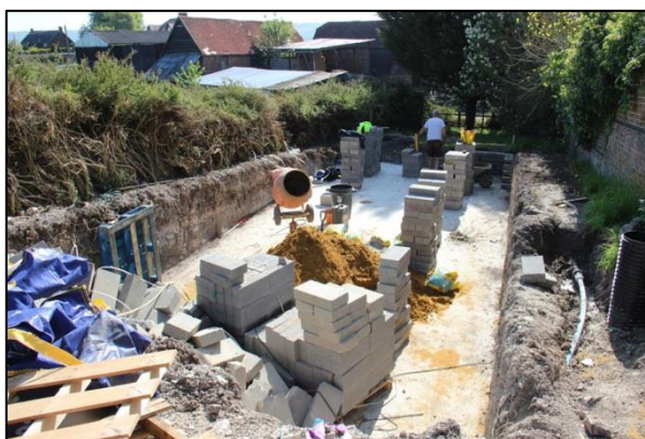
Plate 7: Swimming pool, general area
