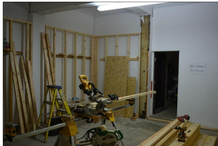
Plate 3: Northwest corner of the shop showing the frame for the new wall and ceiling lining
