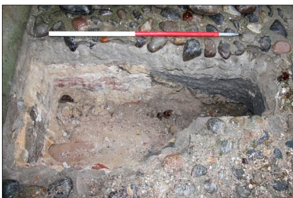
Plate 28: Service trench to the north of the porch including stone and brick foundation [201], view west
