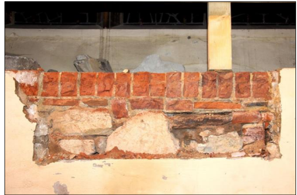
Plate 33: Brickwork beneath plaster in the west wall of the porch, view west
