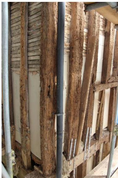
Plate 72: Timbers at southern corner of the first floor
