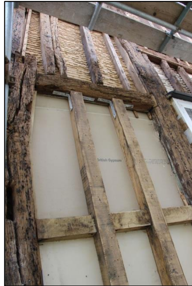
Plate 65: Timbers to the north of the first floor window
