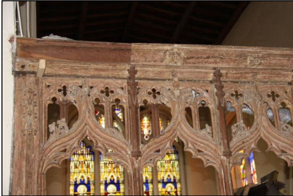
Plate 58: Chancel screen detail showing later repair
