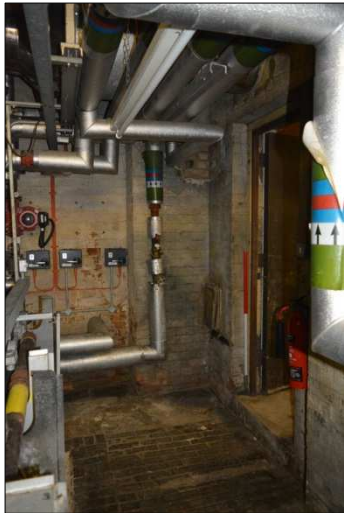
Plate 29: Room B3: boiler room looking west (22)
