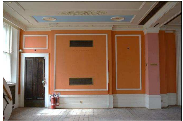
Plate 60: G2b: south wall detail (6)
