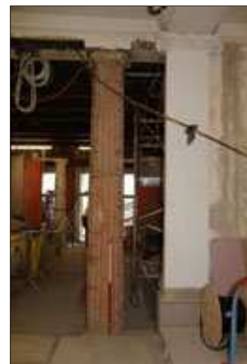
Plate 87: G3: stripped column (53)
