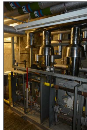
Plate 28: Room B3: boiler room looking east (21) (41)
