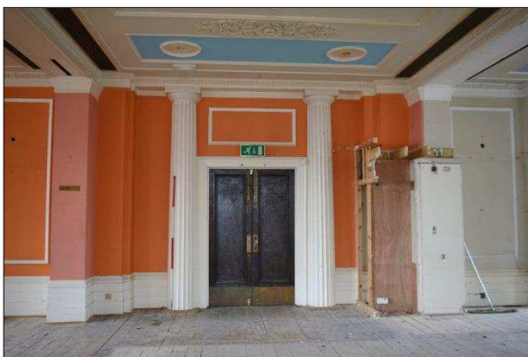
Plate 61: G2b: south wall detail (7)
