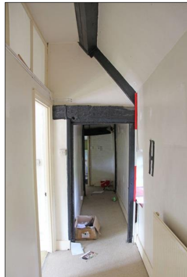
Plate 10: Truss 2, facing west (5)
