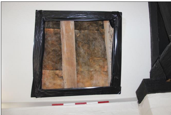
Plate 29: Exposed rafters adjacent to Truss 3, facing south (28)
