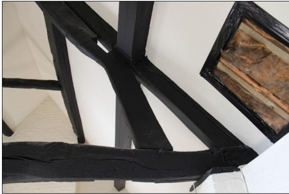
Plate 19: Truss 3, facing west (8)
