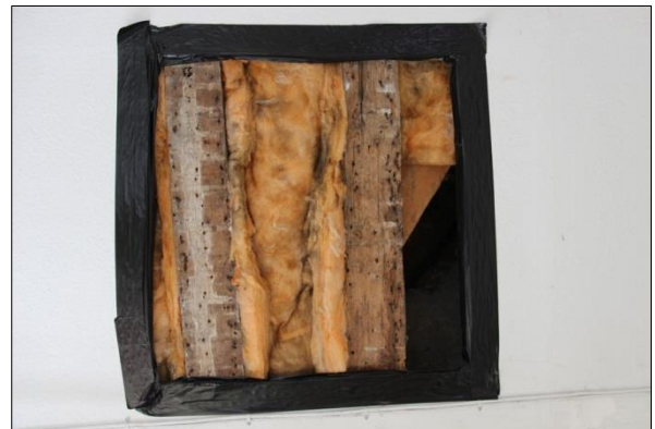
Plate 30: Exposed rafters adjacent to Truss 3, facing north (32)
