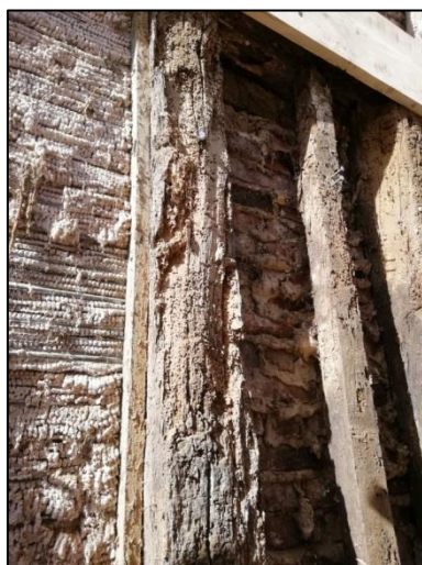
Plate 50: Decayed stud with modern plasterwork to the left
