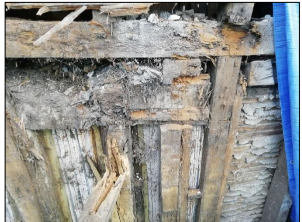
Plate 49: Decay to 18 th century frame
