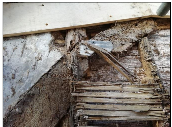
Plate 35: East wall: decayed brace & stud with laths to front and modern plasterwork to rear
