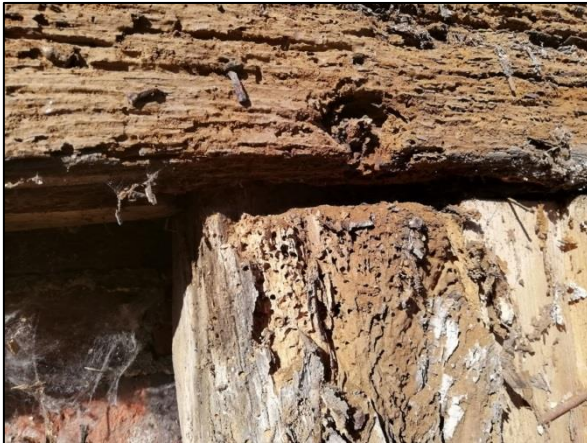
Plate 46: Detail of decay to post and beam
