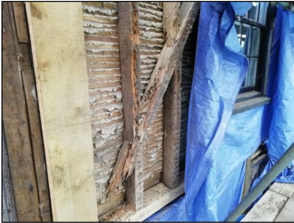
Plate 10: North wall: first floor east brace
