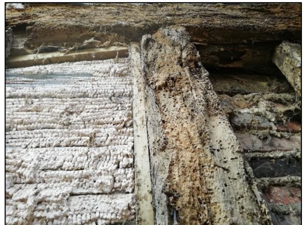
Plate 39: East wall: plasterwork to left of original stud and brickwork to the right
