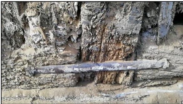
Plate 48: Iron tie holding decayed post and beams
