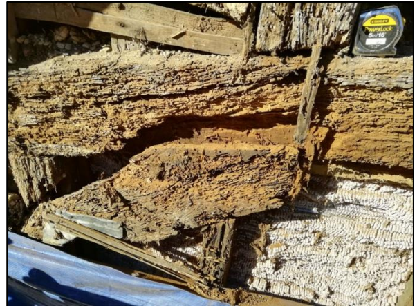
Plate 47: Detail of decay to beam and brace
