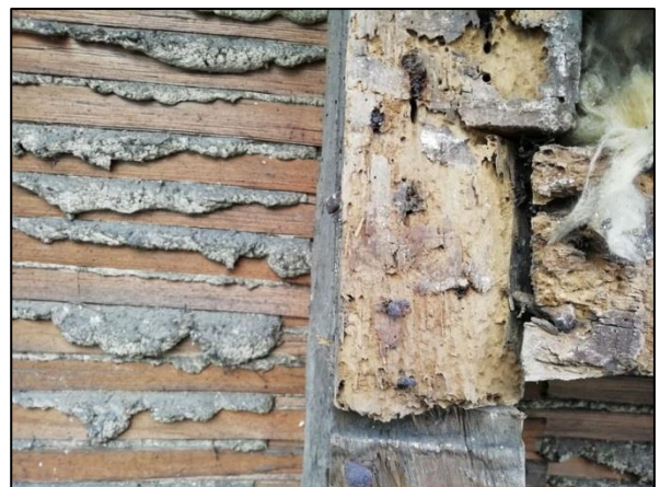
Plate 51: Decayed post with lath & plaster behind
