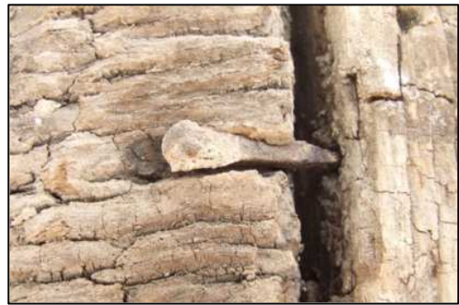
Plate 26: South elevation: nail used to fix rail to studs
