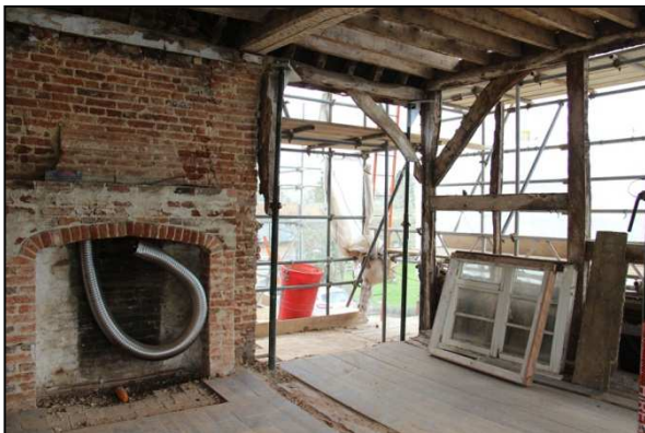
Plate 37: North east corner
