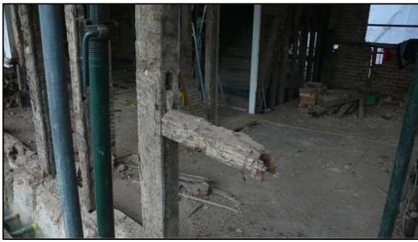
Plate 19: South elevation: detail of decayed rail
