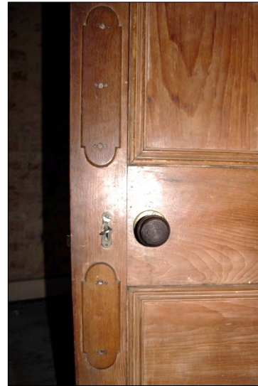
Photo G16: G1: wooden finger guard mounts on door to G5
