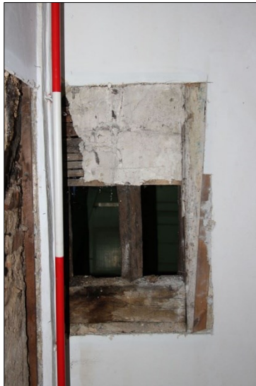
Photo F83: F15: detail of timber work in east wall, mullion window from F11
