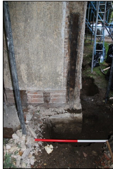
Plate 3: French drain at the northeast corner showing timber frame above the footing
