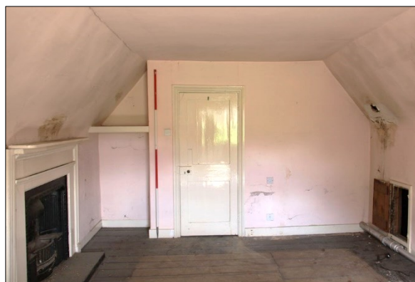
Photo S16: S5: north wall
