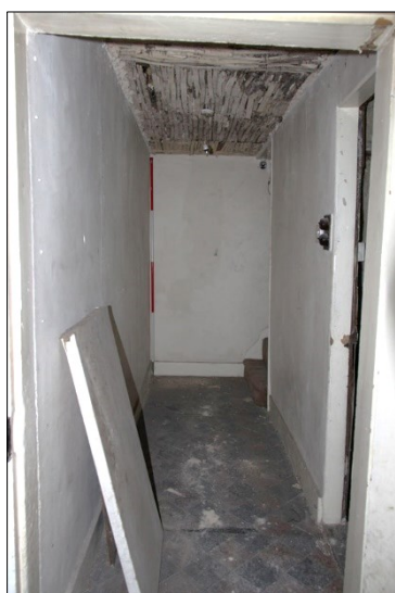
Photo G84: G12: facing east, basement stairs on near right, stairs to first floor on right at far end
