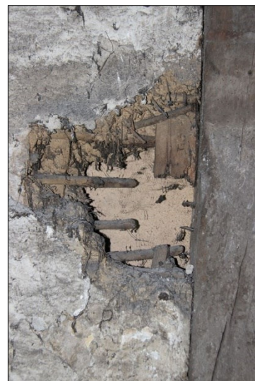
Photo F65: F11: wattle and daub below window
