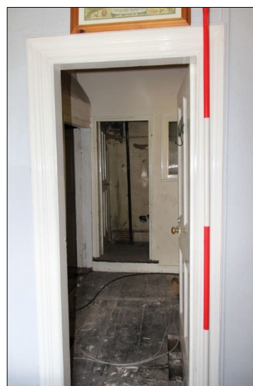
Photo F74: F12: view across F12 from F13 towards F14, facing north
