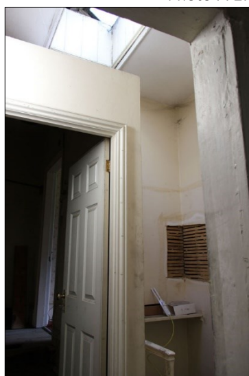
Photo F73: F12: partition wall dividing Northside and Abdale House, facing southeast
