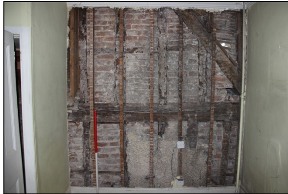
Photo F39: F5: north wall stripped exposing timber frame from east cross wing
