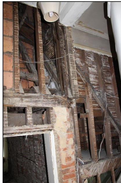
Photo F12: F1: Wall and roof timbers viewed from east end of F1
