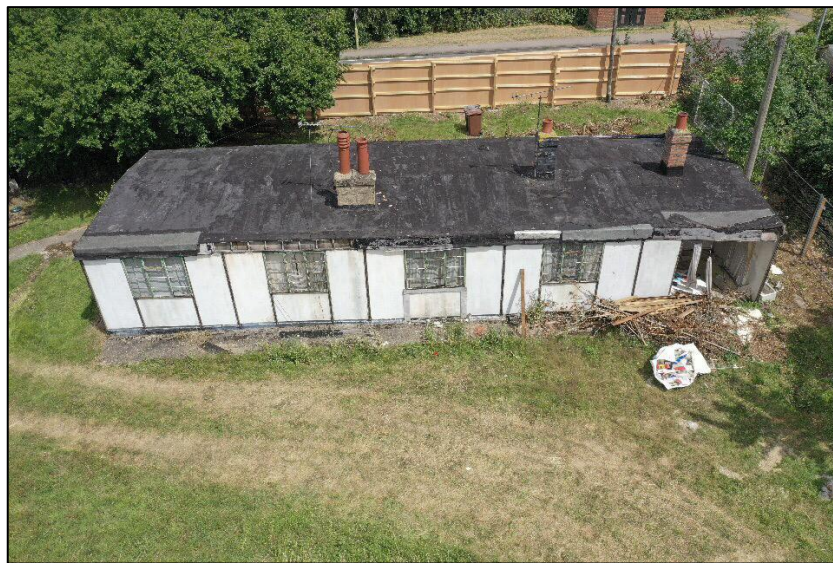
Figure 3: Front and rear elevations taken before the roof was removed (Courtesy of Griggs)
