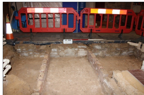
Plate 15: North section of excavation, south aisle; note the two rows of brick
