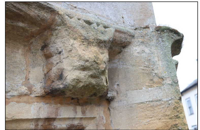
General erosion (Carstone)
