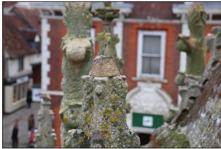
Loss of top of pinnacle
