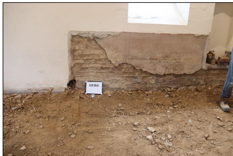
Plate 4: Detail of the south wall showing the old and new render over the brickwork and the date 1985
