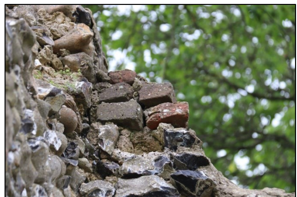
Shot 66: Brick repairs at the top of the freestanding section of south wall
