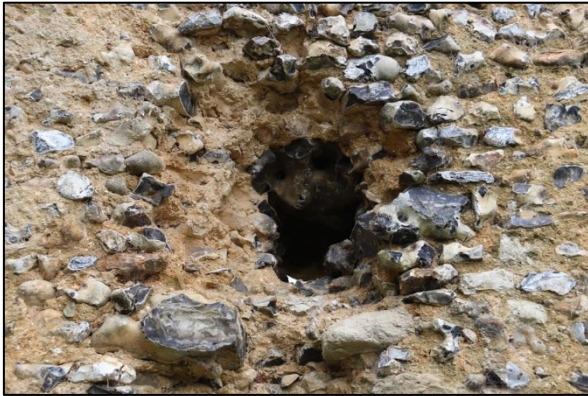
Shot 57: Putlog hole with no lintel in west wall (west wall middle level)
