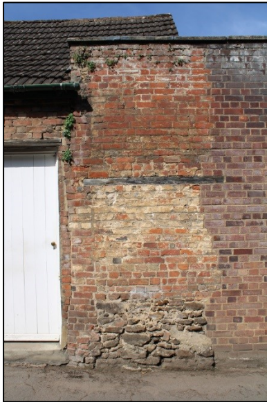
Plate 33: Former boundary wall/flat roofed section, remains of earlier boundary wall, detail of facing west
