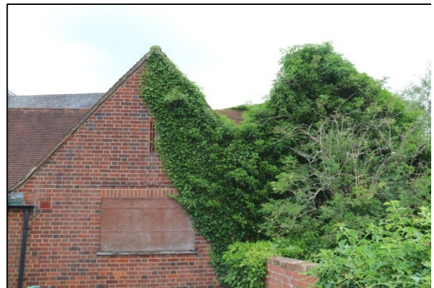
Plate 46: The Old Telephone dual pitched slated roof (adjacent to southern boundary wall), facing east
