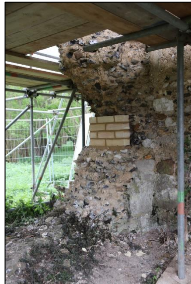
Plate 12: West side of south nave wall opening with sample brickwork from the northeast
