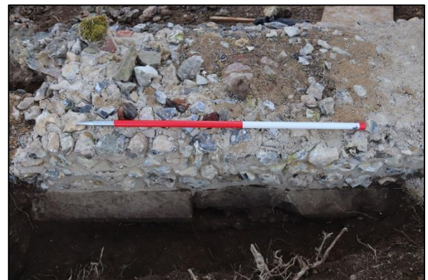
Plate 26: Detail of moulded stones from the north in the north nave wall
