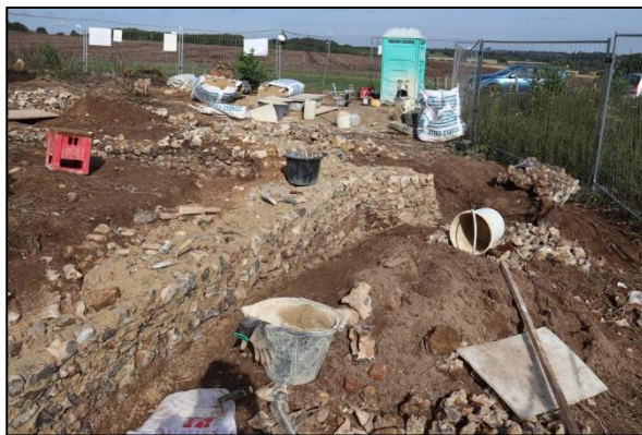
Plate 9: East wall and northeast buttress remains from the south
