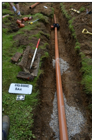
Plate 10: Soakaway 4 service, looking west
