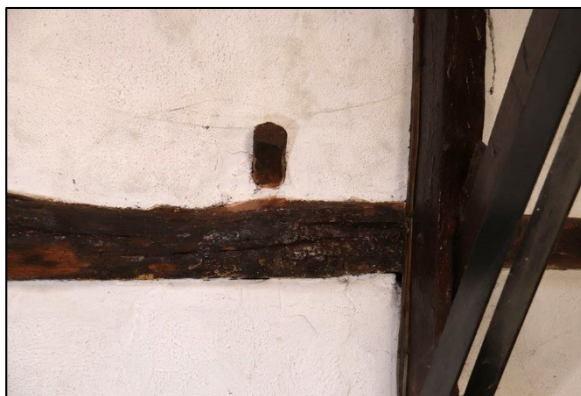
Plate 23: G1: timber detail (south wall)
