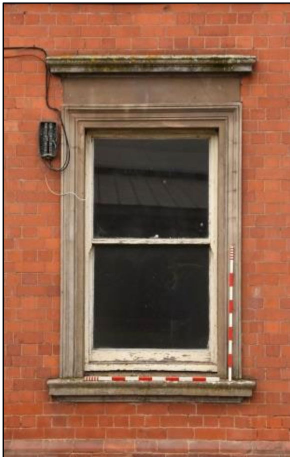
Example of sash window on the 1890s range, taken from the east Fig 26
