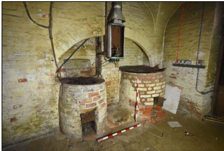
Brick coppers on the south wall of the Scullery, taken from the north-west 136
