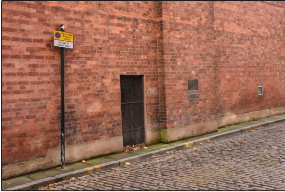
Door giving access to lower ground floor along the western elevation, taken from the north-west Fig 36
