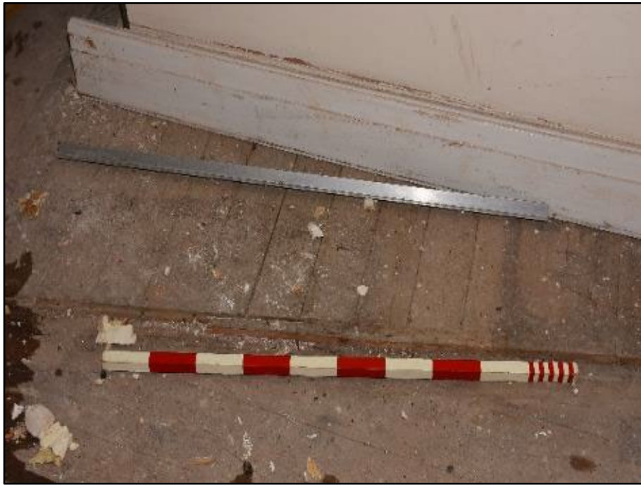
Section of floorboards in the Former Bar Store, taken from the east
