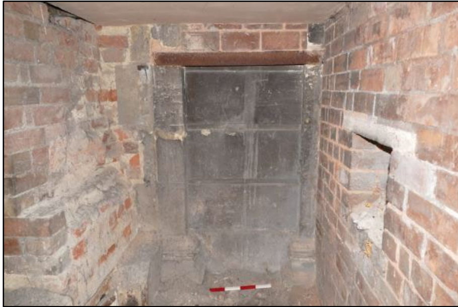
West wall of the void beneath the Portico, taken from the east Fig 151
