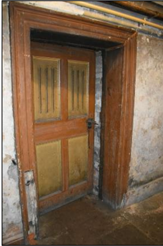
Example of the common door type in the Corridor, taken from the south-west Fig 128
