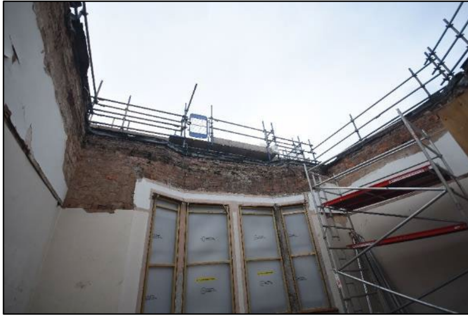
Exposed brickwork to the wall during the monitoring works, looking east Fig 116
