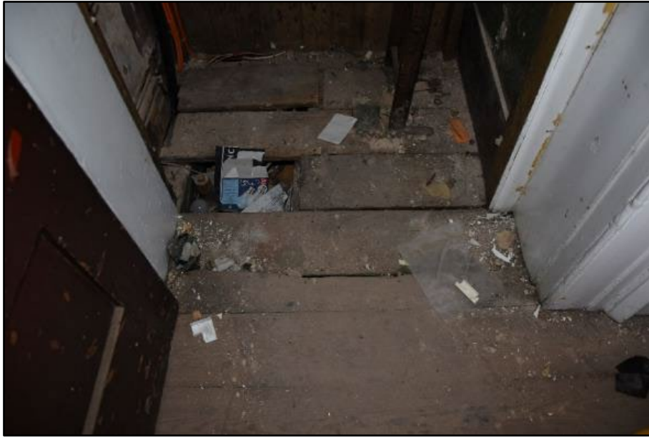
Floorboards in the Central Corridor and service cupboard, taken from the west Fig 52
