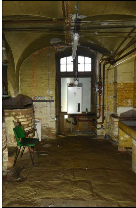
Door to the exterior from the Scullery, opening into the push-out on the south rear elevation, taken from the north Fig 137
