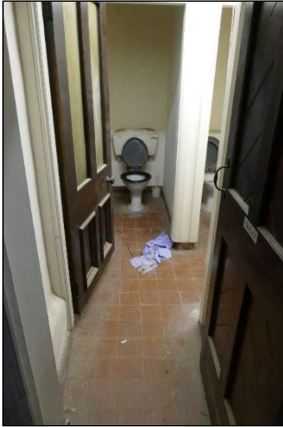
Interior of the WC block within the Summoner's House, looking south Fig 177
