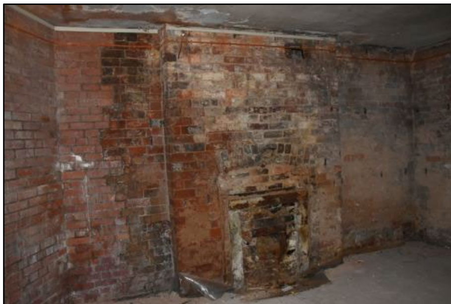
East wall of the Coachmen's Waiting Room, taken from the north-west Fig 162
