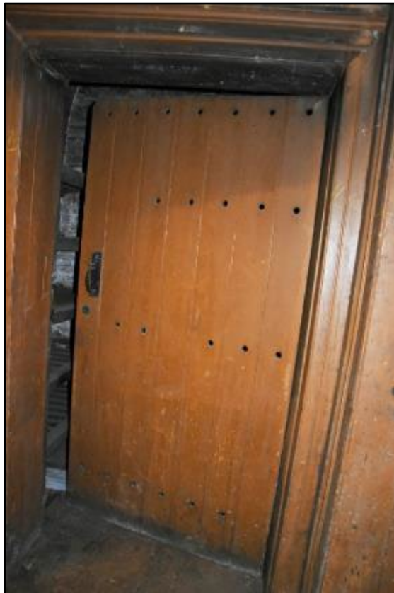
Door to the Wine Cellar from the Corridor, taken from the north Fig 129
