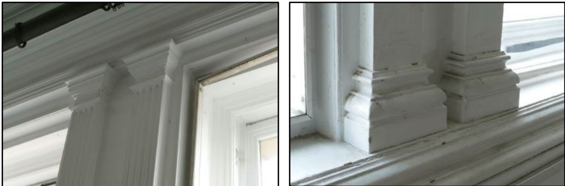
Detail of the sash windows inserted in the 1860s, taken from the south Fig 61
