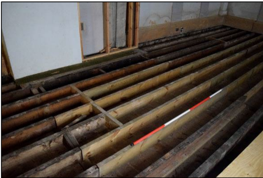
Area of replaced floor joists in the Tea Room, taken from the south-east Fig 65
