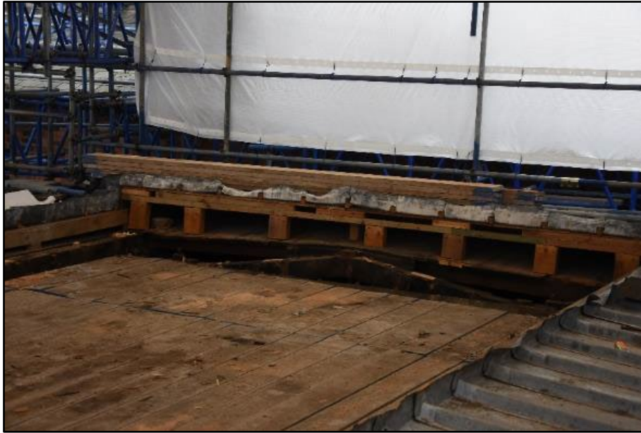
Area of exposed timber frame to the roof lantern above the Tea Room, looking south-east Fig 40
