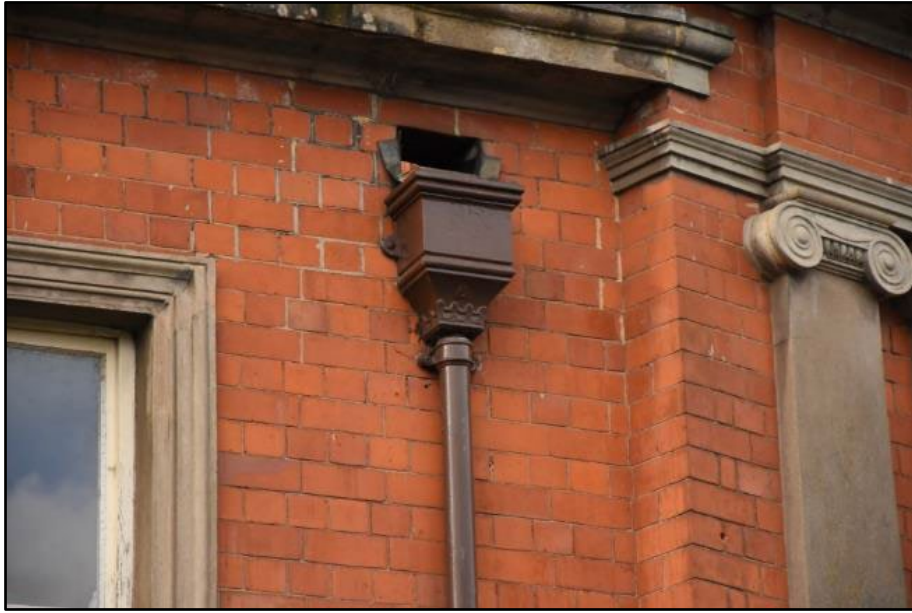
Rainwater hoppers on the elevation of the Summoner's House, taken from the east Fig 27
