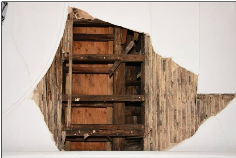
Lath and plaster ceiling revealed in the Central Corridor during monitoring works Fig 53
