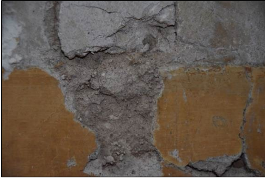
Detail of the plaster to the north wall of the East/West Corridor, taken from the south Fig 94
