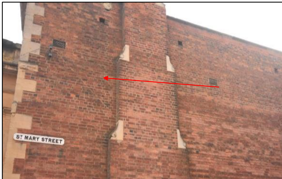
Scar of previously abutting building visible on the west elevation, taken from the north-west Fig 37
