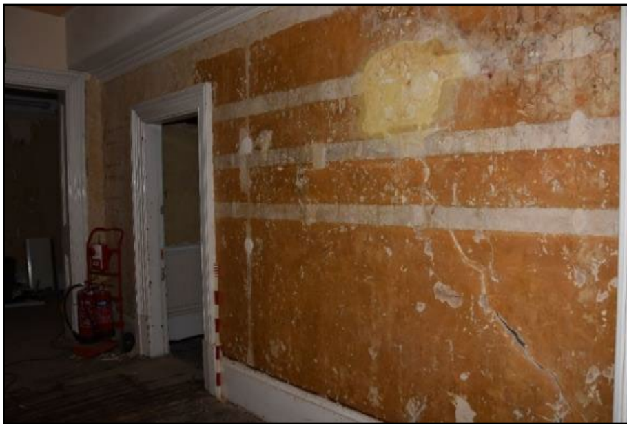
North wall of the East/West Corridor (15) showing line of differing coloured plaster, taken from the east Fig 95
