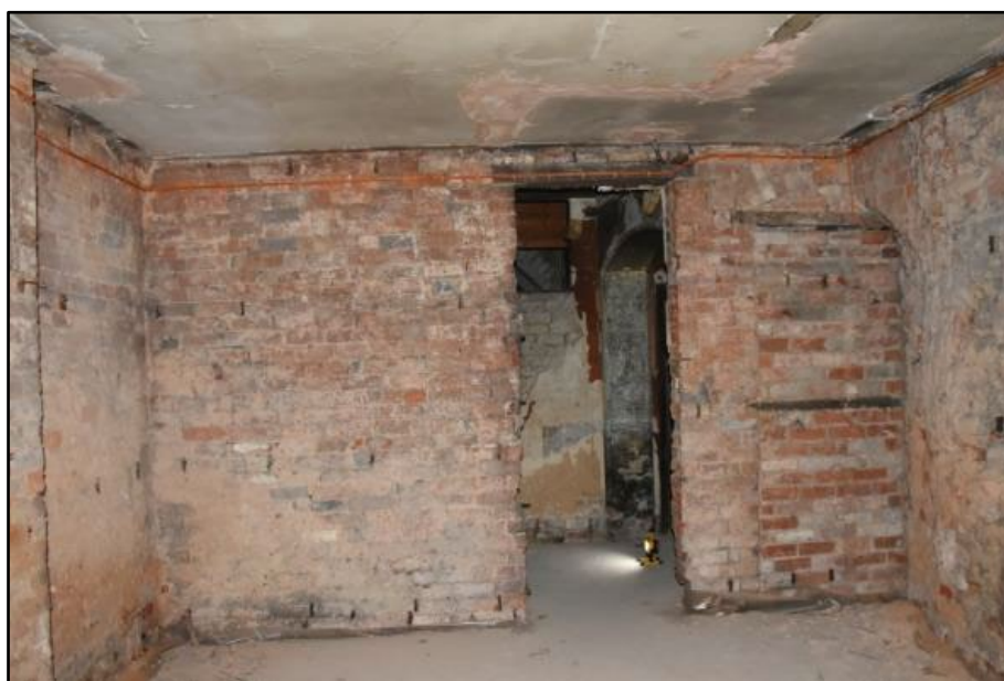
South wall of the Coachmen's Waiting Room, taken from the north Fig 163
