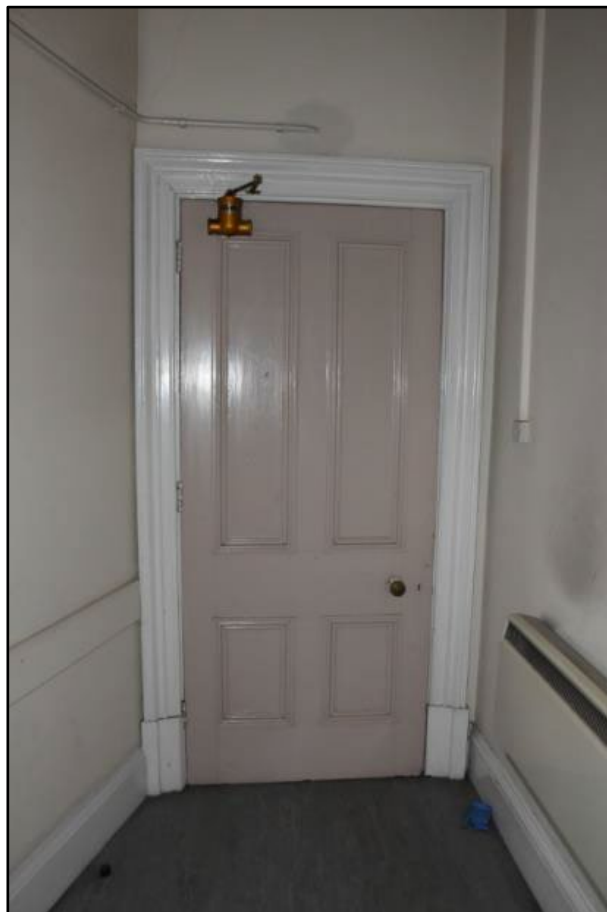
Rear of the door giving access into the Former Restrooms, taken from the north Fig 102
