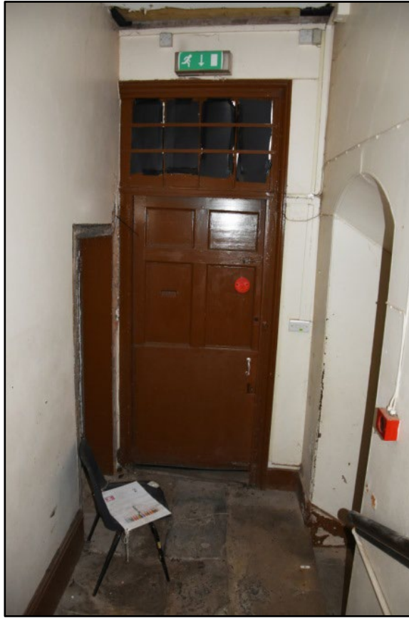
Entrance lobby from the rear of the building, taken from the north Fig 123
