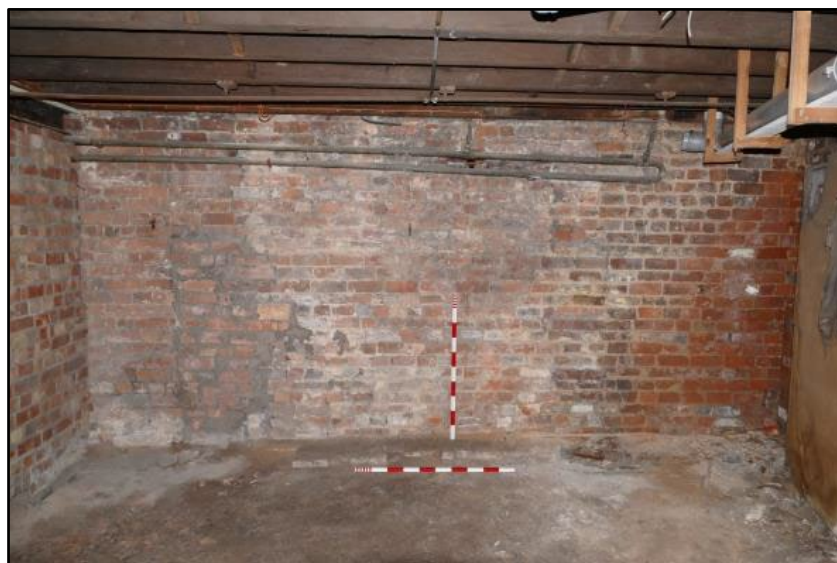
South-east wall of the Coachmen's Waiting Room, taken from the west Fig 170
