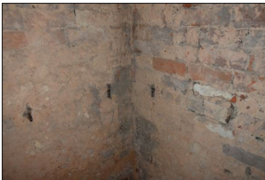
Timber bearers present in the walls in the Coachmen's Waiting Room, taken from the north-west Fig 165
