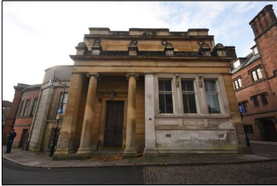
The north elevation of the 1830s range, taken from the north Fig 15
