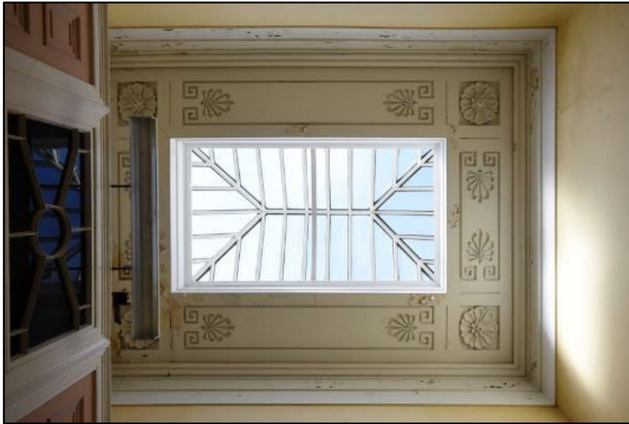
View of the ceiling of the Vestibule and Lobby, taken from the north Fig 44
