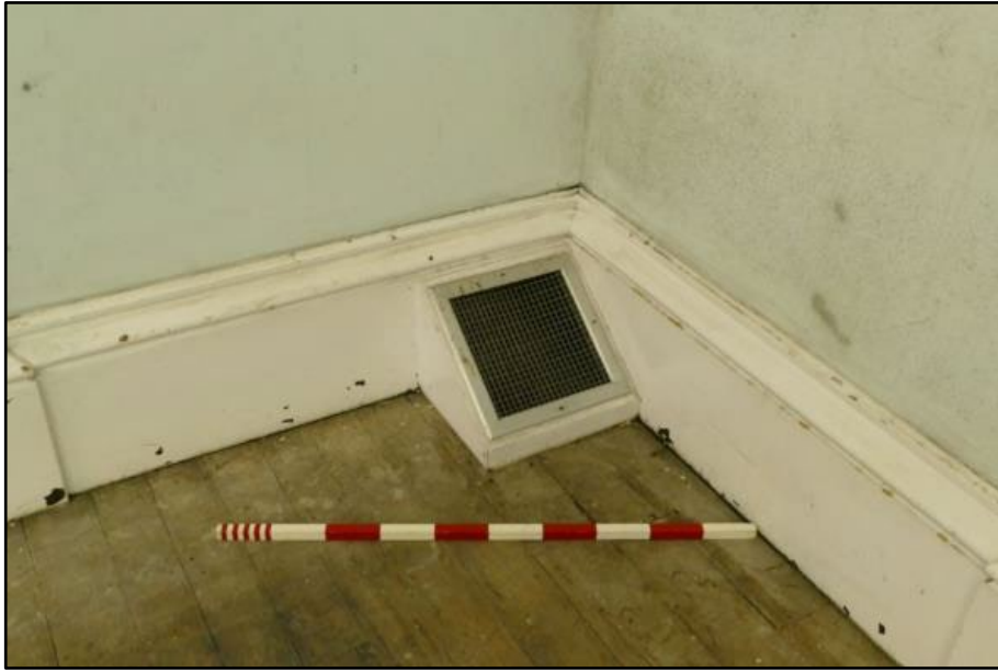
Air vent in the south-east corner of the Tea Room, taken from the north-west Fig 64
