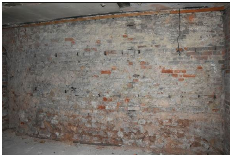
West wall of the Coachmen's Waiting Room, taken from the north-east Fig 164
