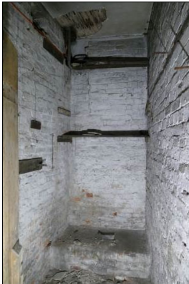
Interior of the Store, directly off the Basement Corridor, looking east Fig 157
