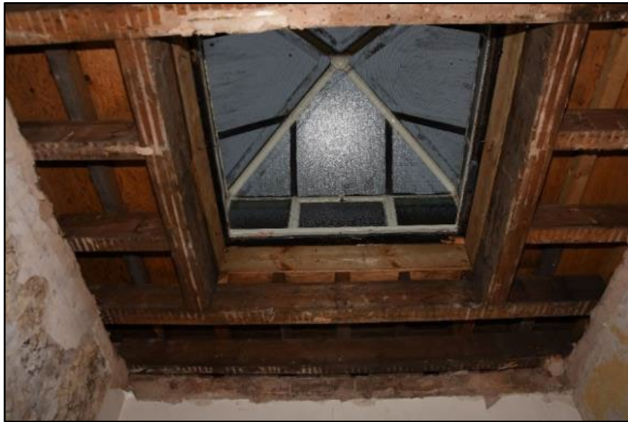
Exposed construction of the ceiling over the eastern section of the East/West Corridor, taken from the west Fig 96
