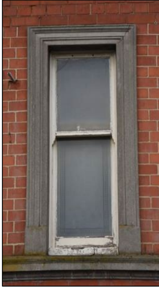
Example of sash window on the 1890s range, taken from the north-east Fig 23
