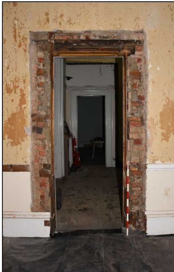
Door frame exposed during the planned works, taken from the east Fig 101
