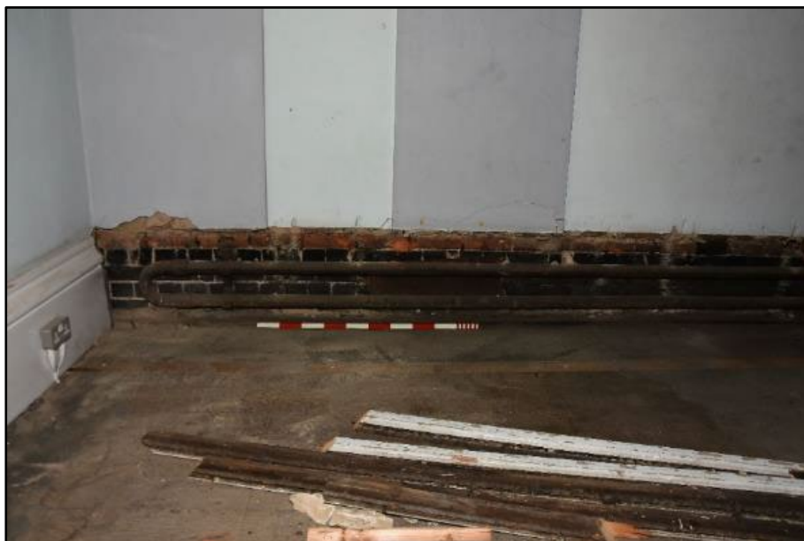
Section of exposed brickwork to the south wall, taken from the north Fig 82
