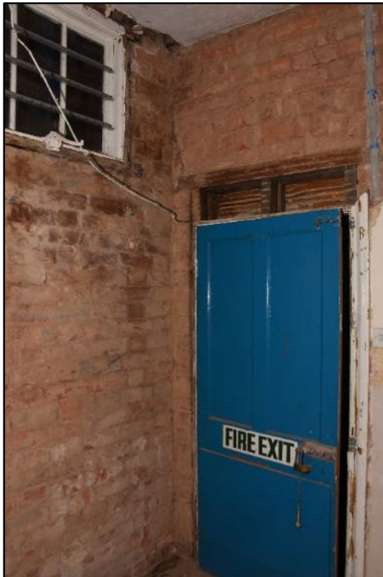
Entrance hall in the Summoner's House stripped during monitoring phase, looking south-west Fig 176
