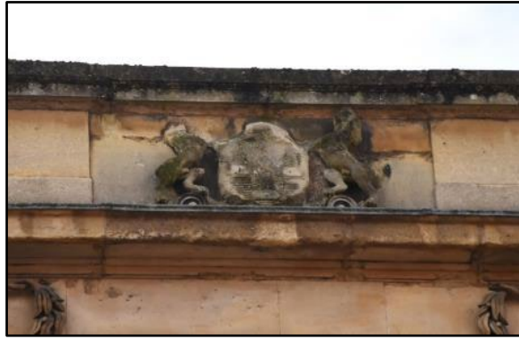
Architectural details on the 1830s north elevation, taken from the north Fig 18
