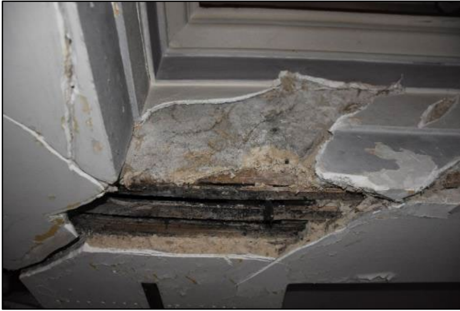
Cracks in the plasterwork to the lanterns frame reveal laths beneath, looking west Fig 80
