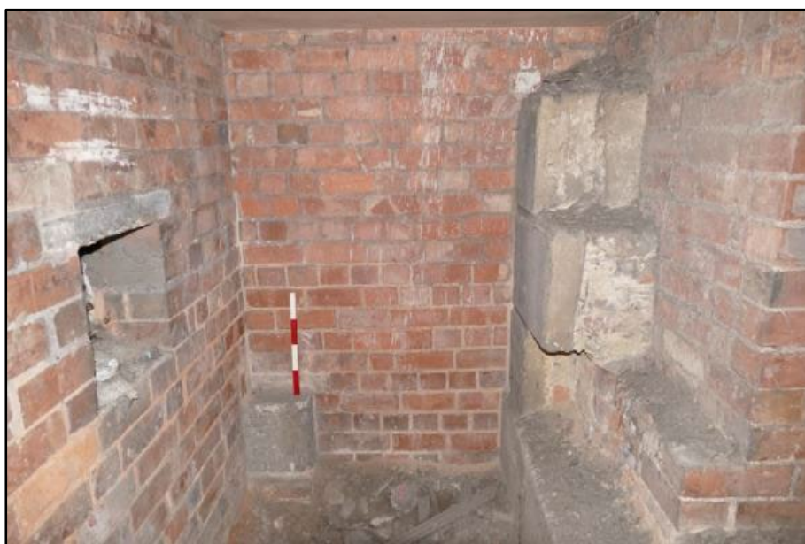
East wall of the void beneath the Portico, taken from the west Fig 150
