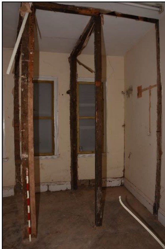
Internal partitions to the WCs during monitoring of works, taken from the south-west Fig 104
