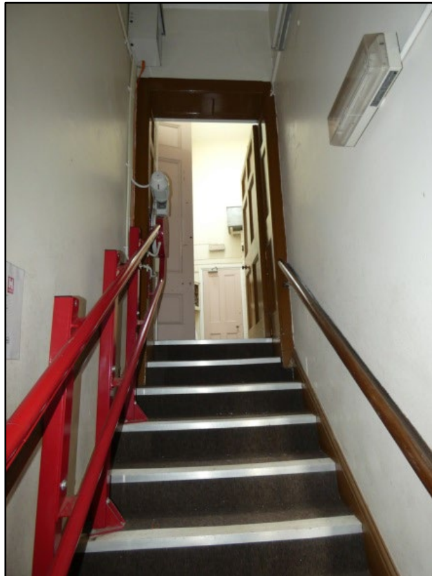
Stairs from ground floor to lower ground floor, taken from the south
