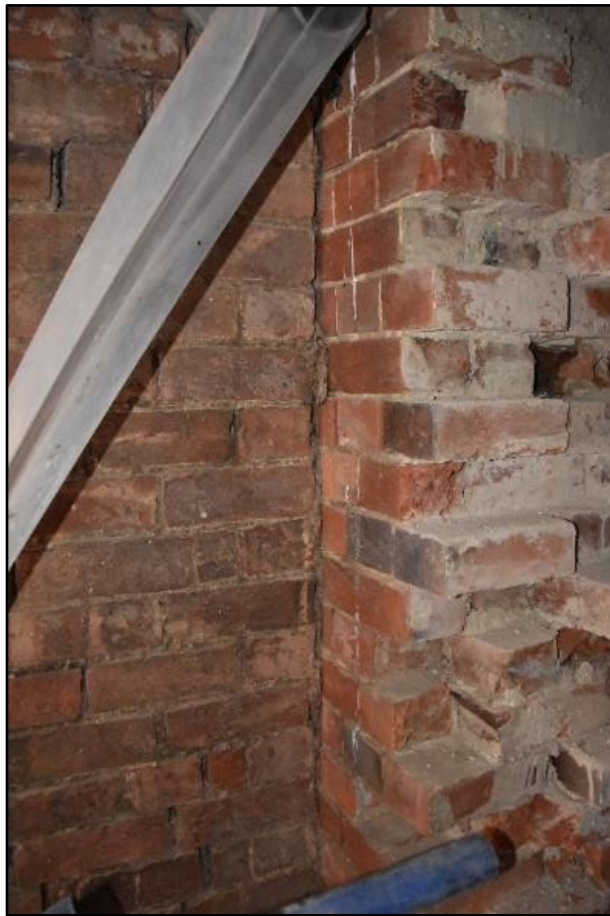
Brick walls of the porch (left) and ballroom (right), looking south-west Fig 31
