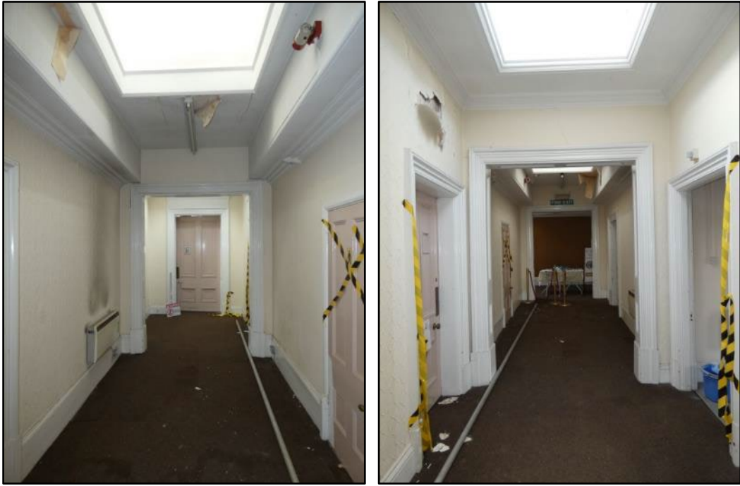
View of the East/West Corridor, western section (left) taken from the west and eastern section (right) taken from the east Fig 92
