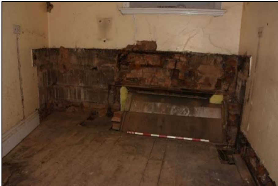
Exposed area of brickwork in the Service area (27), taken from the west Fig 119
