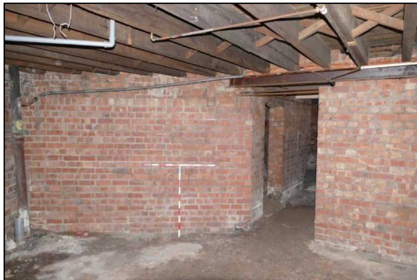
South wall of the Coachmen's Waiting Room, taken from the north Fig 169
