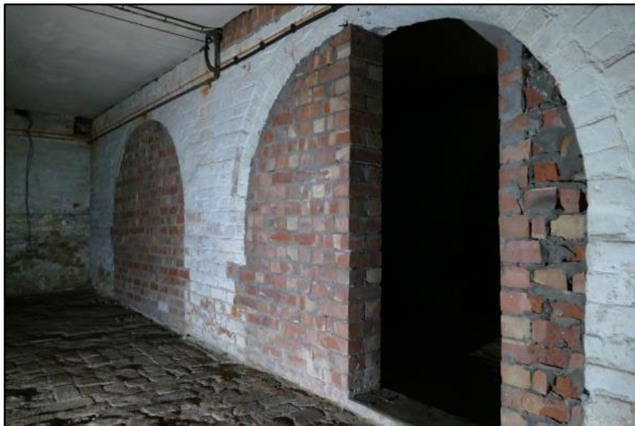
Brick arched partitions in the Stores, later infilled, taken from the south-east Fig 146
