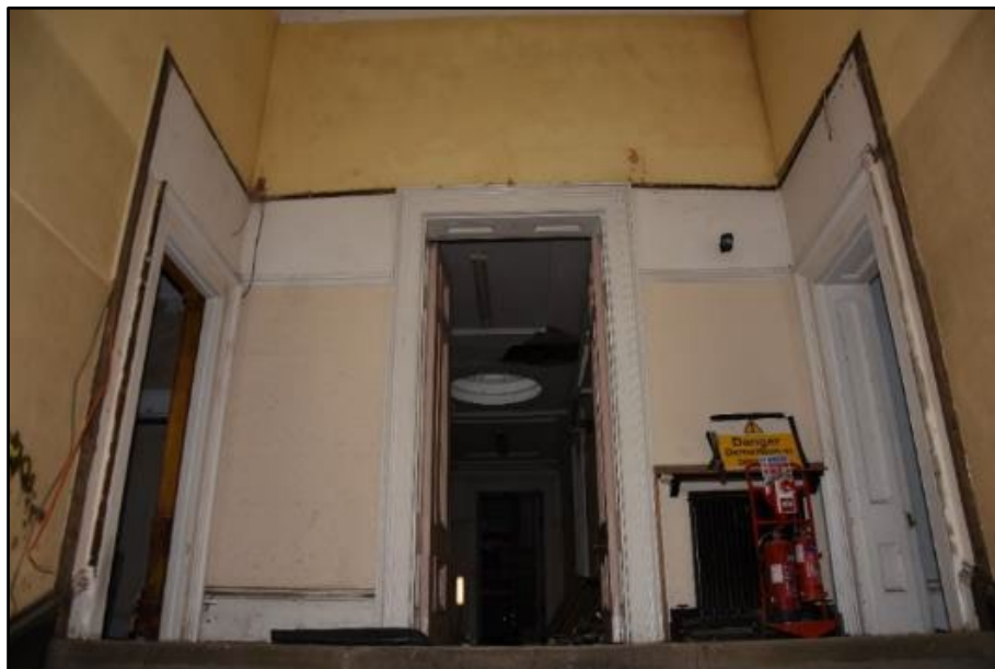
The Lobby after the soft-strip during the planned works, taken from the north Fig 47
