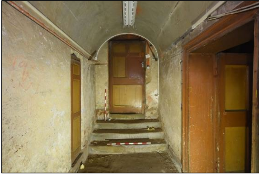
Access from the lower ground floor Entrance Lobby to the corridor, taken from the west Fig 124
