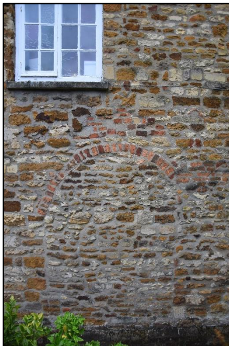
Arched blocked opening to the south elevation of the rear range, looking north Fig 32
