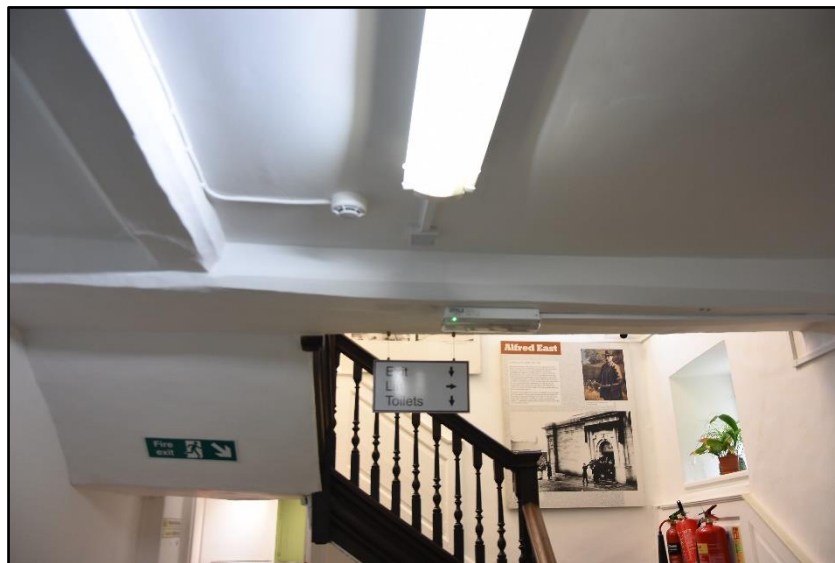
Ceiling joists to the landing in the main range (FF01), looking north Fig 67
