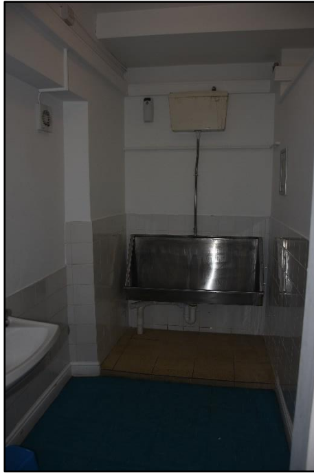
View of the men's WCs (GF05), showing blocked window and chimney stack, looking north Fig 43
