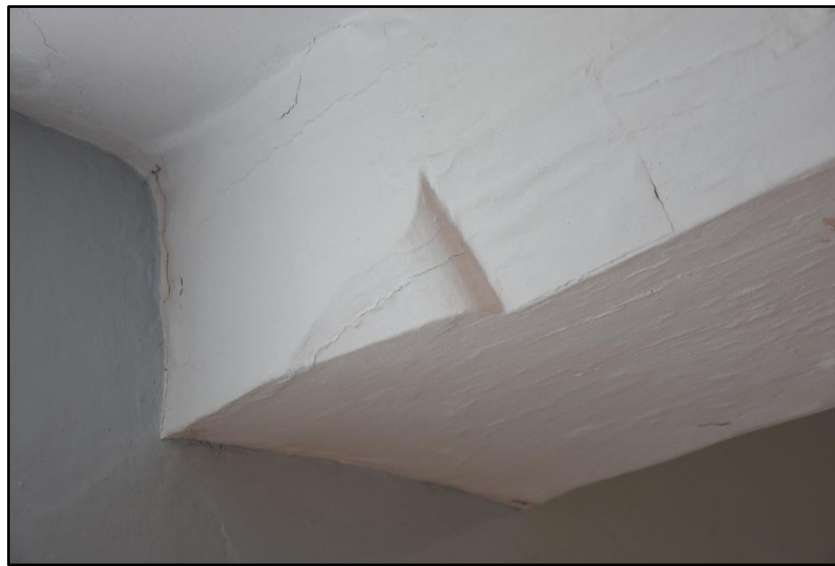
Chamfer and stop to the ceiling beams in FF02, looking south Fig 72
