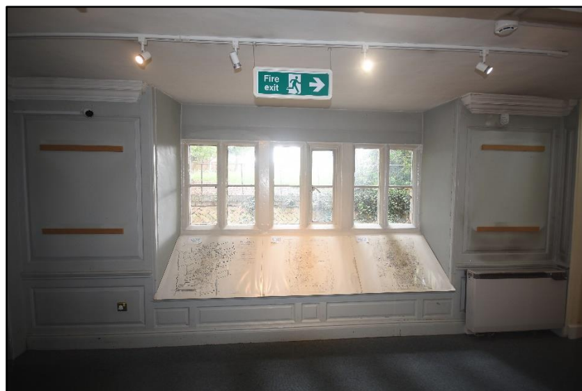
Stone mullion window in the green exhibition room (GF03), looking east Fig 58
