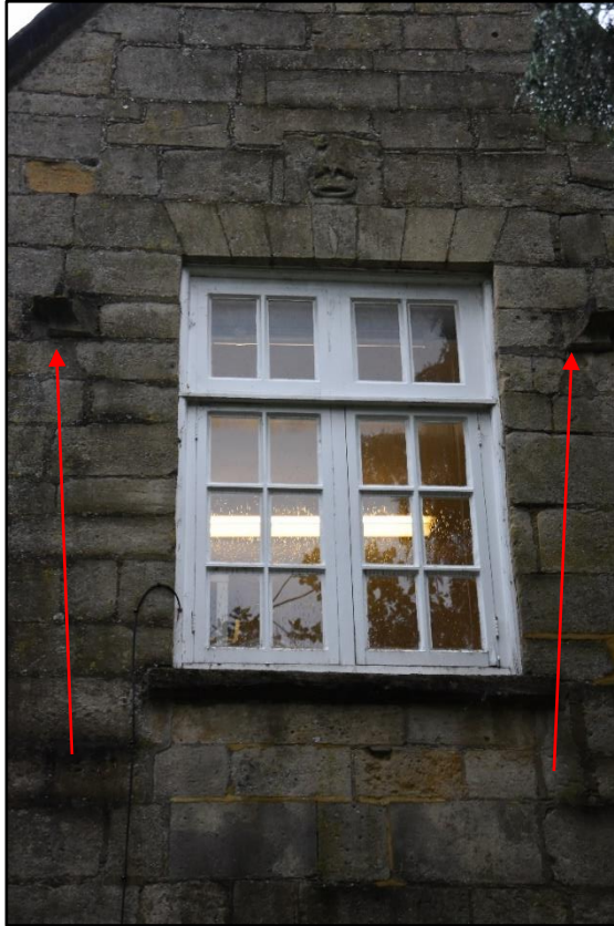
Second floor window to the east elevation of the rear range, label stops indicated, looking west Fig 28
