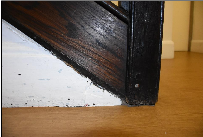
Detail of the carpentry to the newel post of the staircase in GF01, looking east Fig 49
