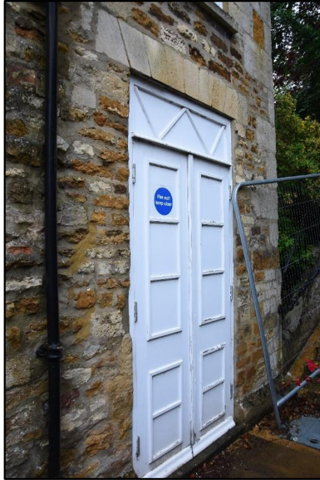
Fire door to the south elevation of the rear range, looking north-east Fig 33
