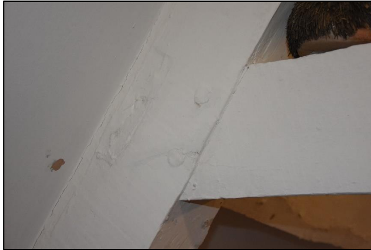
Empty mortise to the east face of the truss in the roof over the rear range, looking west Fig 95
