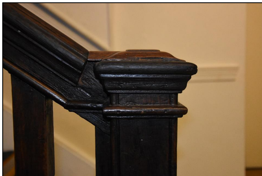
Detail of the newel post to the staircase in GF01, looking east Fig 48
