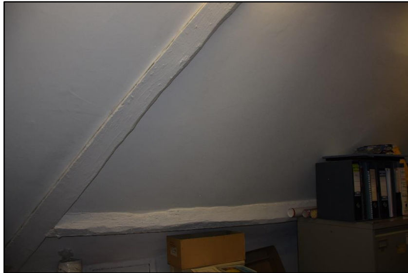
Hip rafters in the roof over the main range, looking west Fig 91
