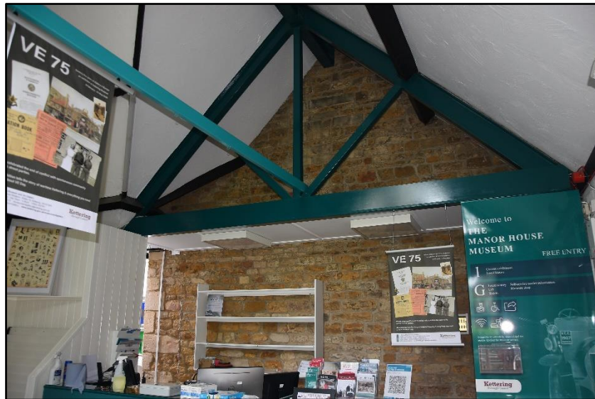
Exposed north formerly external wall of the north range within the museum range (GF06), looking south-east Fig 64
