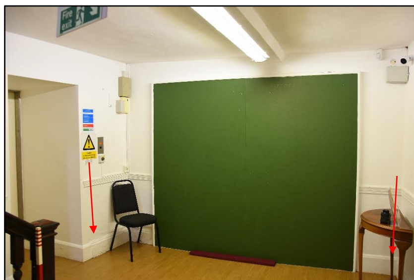
View of the stair hall (GF01) and the breaks in skirting indicated, looking south-east Fig 46
