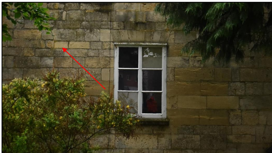
First floor window to the east elevation of the rear range, area of interest indicated, looking west Fig 27
