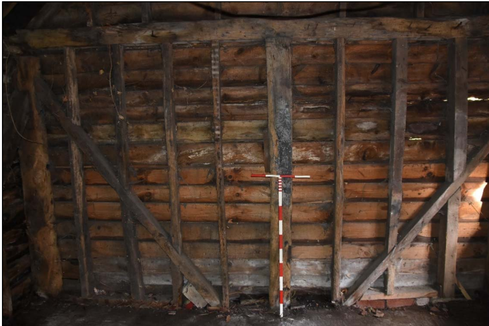
Timber studwork to the north wall of Store D, looking north-west Fig 35
