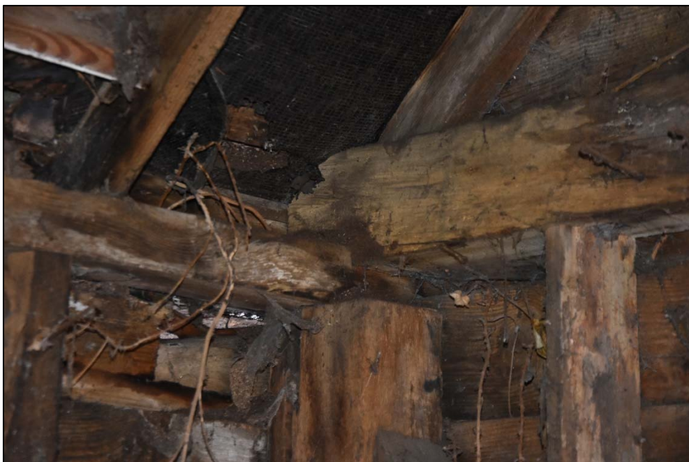
Corner post, wall-plate and tie-beam to the north-west corner of Store D, looking north Fig 34
