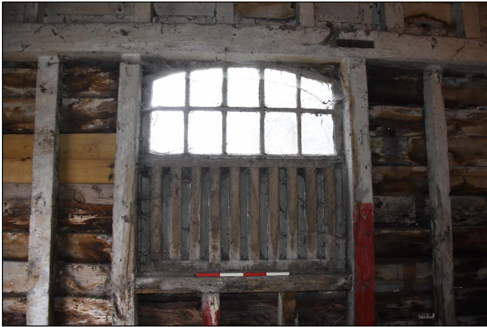
The window to the west wall of Store A, looking north-west Fig 11
