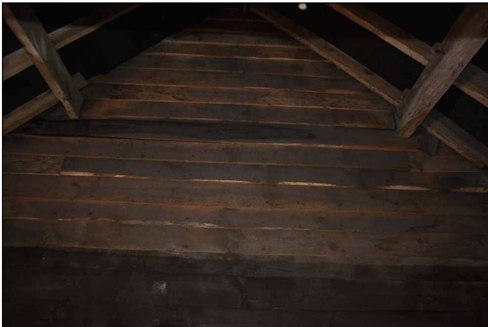
Weather-boarded gable to the south wall of Store D, looking south-west Fig 32
