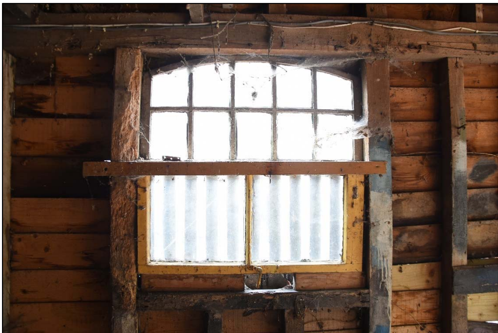
Window in Store C with part of another window inserted over the lower grille, looking north-east Fig 28
