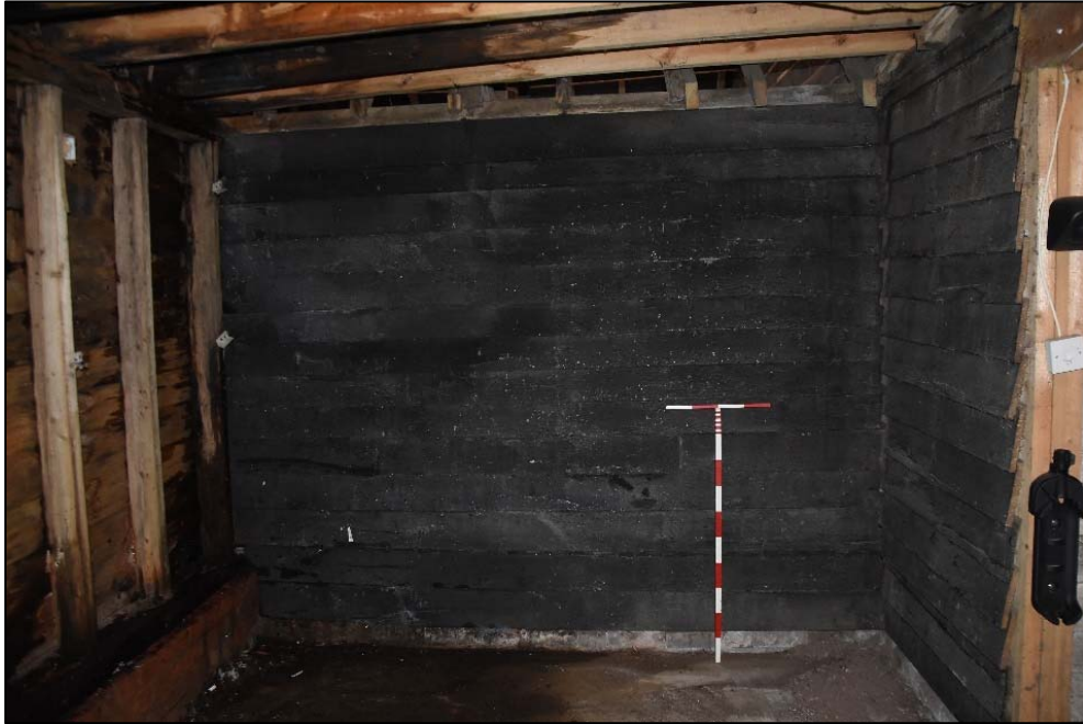
Former exterior weather-boarding to the north range, now housed within Store E, looking east Fig 39
