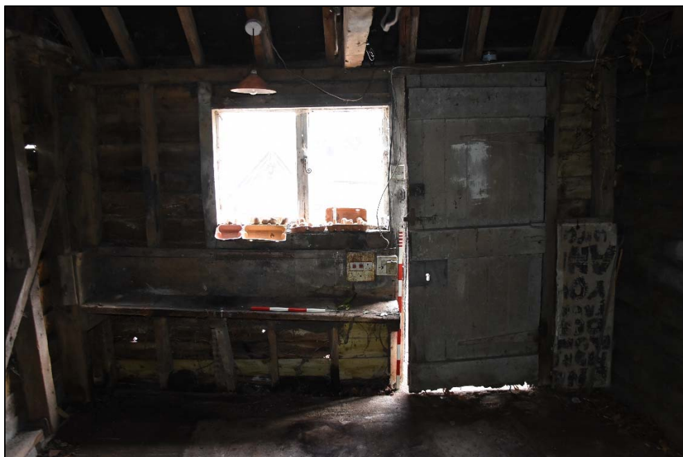
East wall of Store D showing door, window and shelf, looking south-east Fig 30
