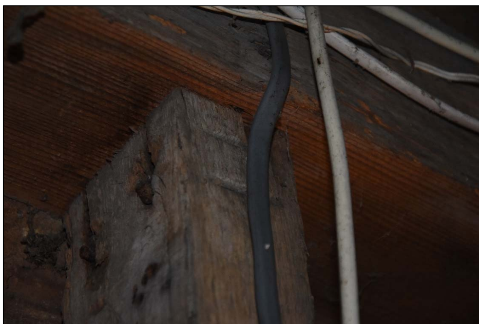
Timber mark at the top of a stud on the west wall, looking north-west Fig 17
