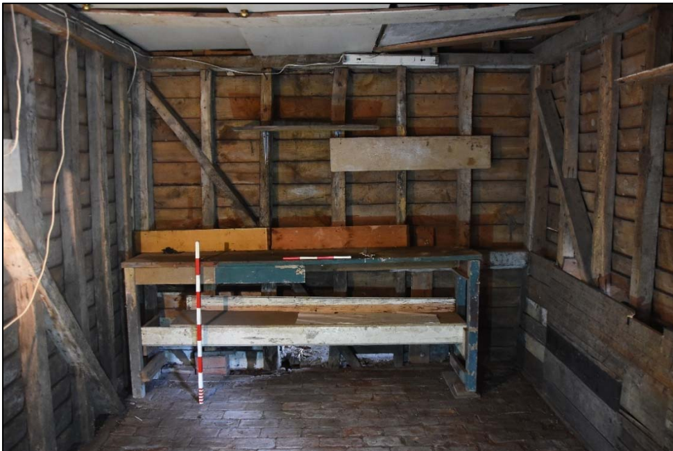
Studwork and shelf to the north wall of Store B, looking north Fig 19
