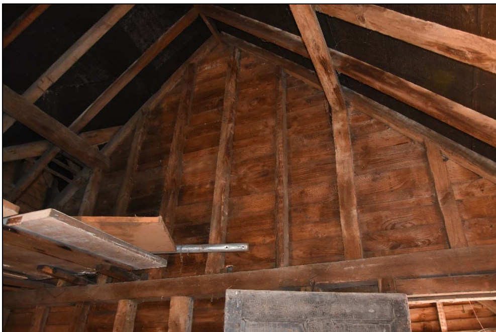
Closed partition above the wall-plate on the east wall of Store B, looking north-east Fig 21
