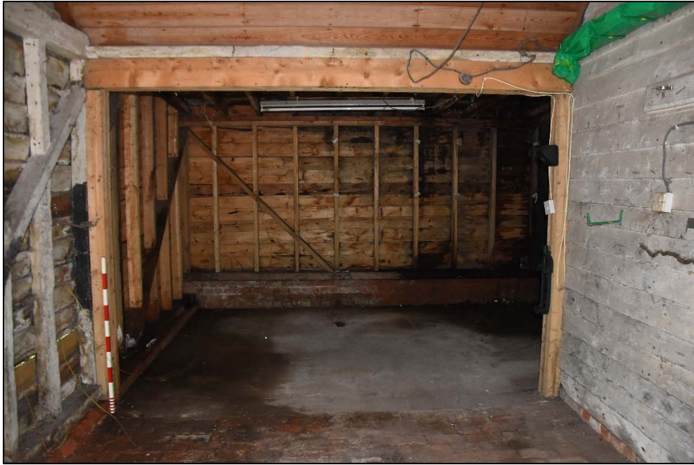
North wall of Store A which has been altered with the addition of Store E further to the north, looking north-west Fig 13
