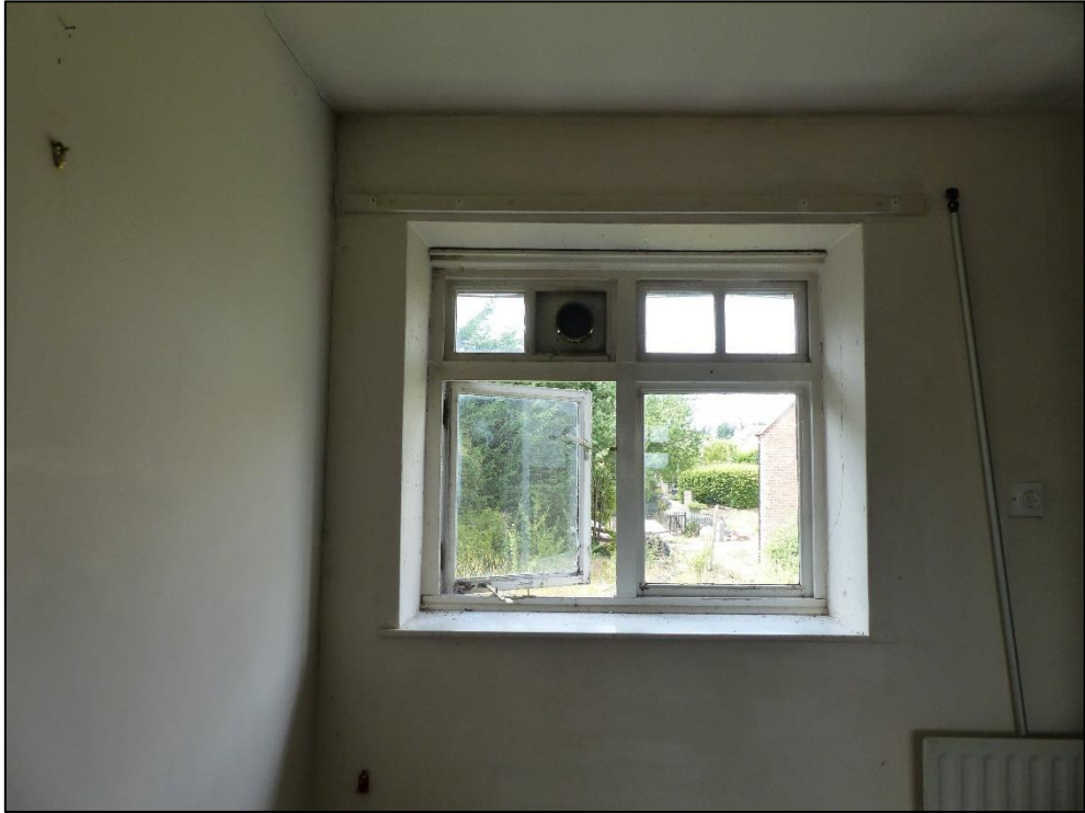
Window to the landing at the north end of the rear corridor (FF06), looking west Fig 85
