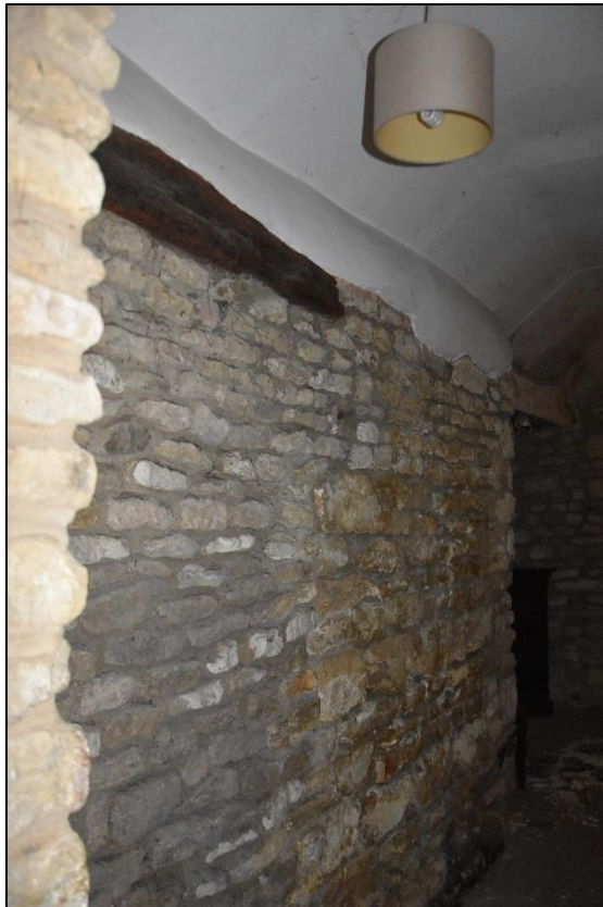
Exposed stone to the north wall of the entrance corridor, looking east Fig 59
