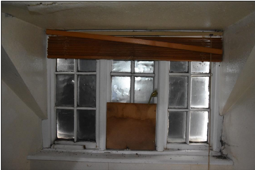
Window within one of the bedrooms to the first floor (FF04), looking south-west Fig 78
