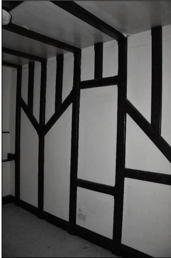
Fictive timber-framing in one of the first floor bedrooms (FF03), looking north Fig 76
