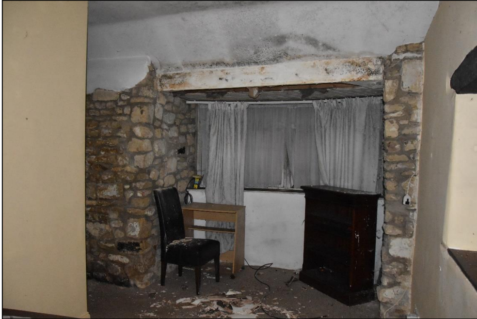
Manager’s flat lounge area (GF22), showing pushed-out bow window, looking north-east Fig 62
