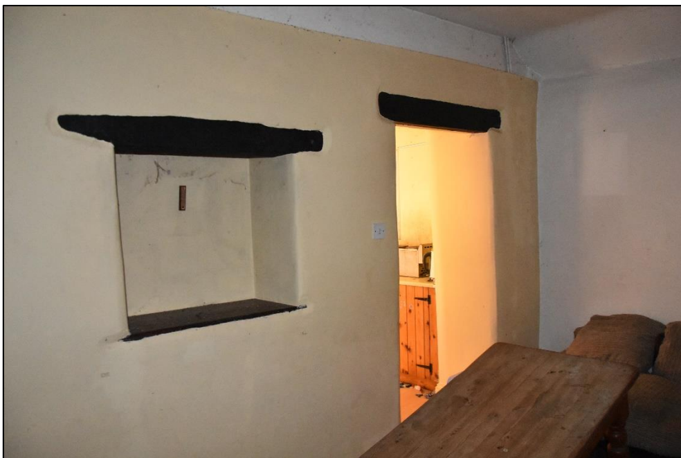
Blocked window and doorway within the Manager’s flat lounge (GF22), looking south Fig 63
