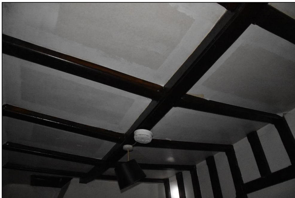
Ceiling joists in one of the first floor bedrooms (FF03), looking north-west Fig 77
