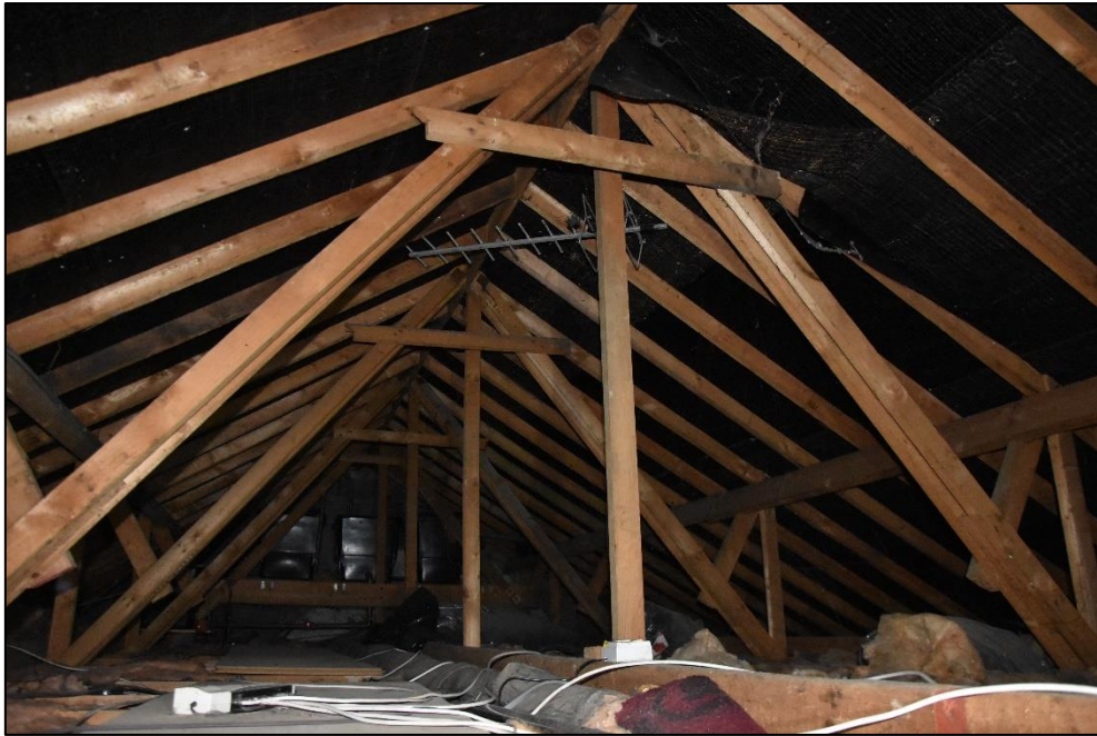
Roof structure over Range 5 visible from a roof hatch at the north end, looking south-west Fig 104
