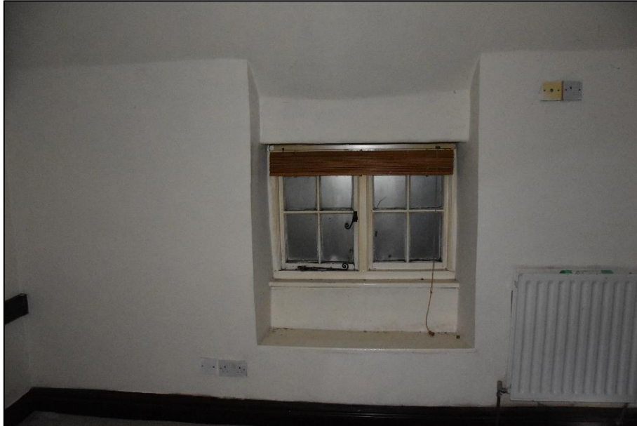
Window to the south wall of a first floor bedroom (FF02), looking south-west Fig 70
