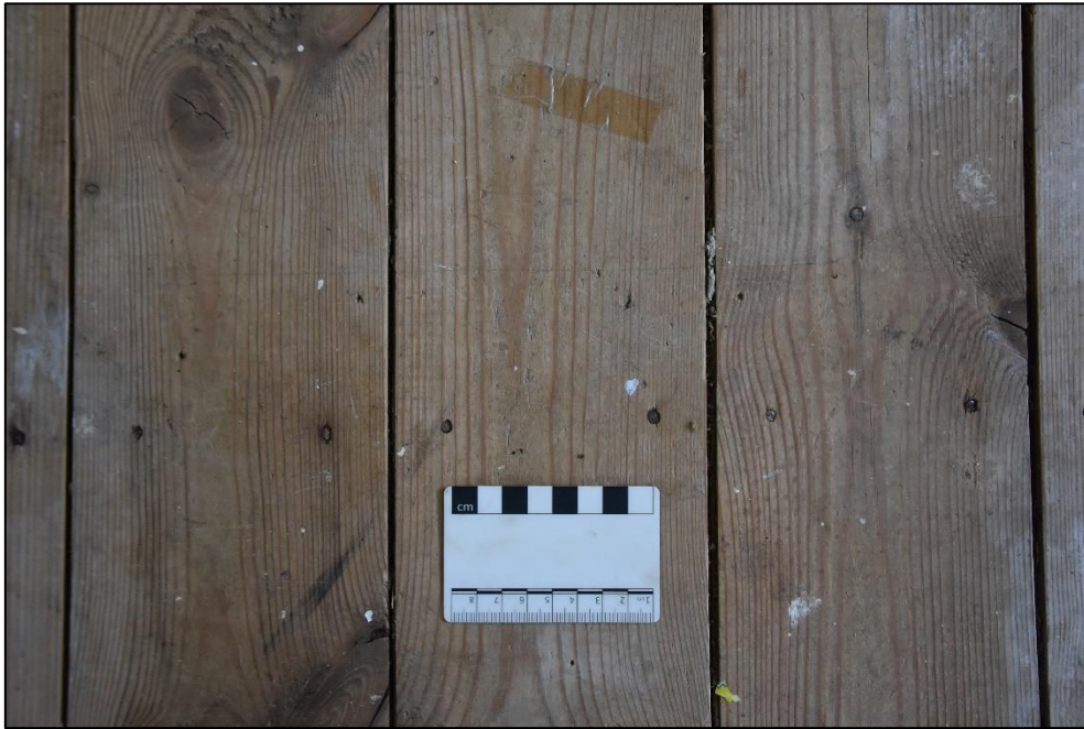
Exposed floorboards to a first floor bedroom (FF10), looking north-west Fig 94
