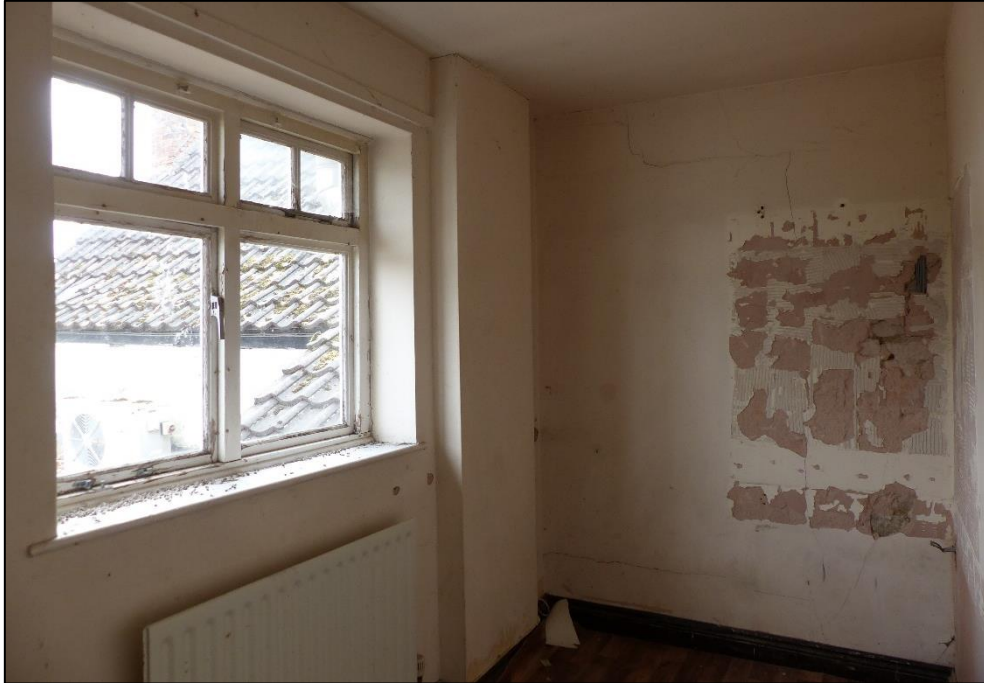
View of room FF11 which may have formerly been a bathroom, looking south-east Fig 96
