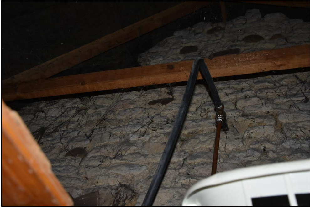
East gable end of Range 3, visible within the roof space, looking north-east Fig 102
