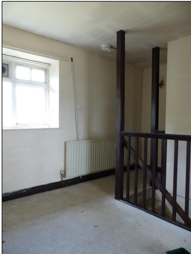
Landing area at the north end of the rear corridor (FF01), looking north-west Fig 86
