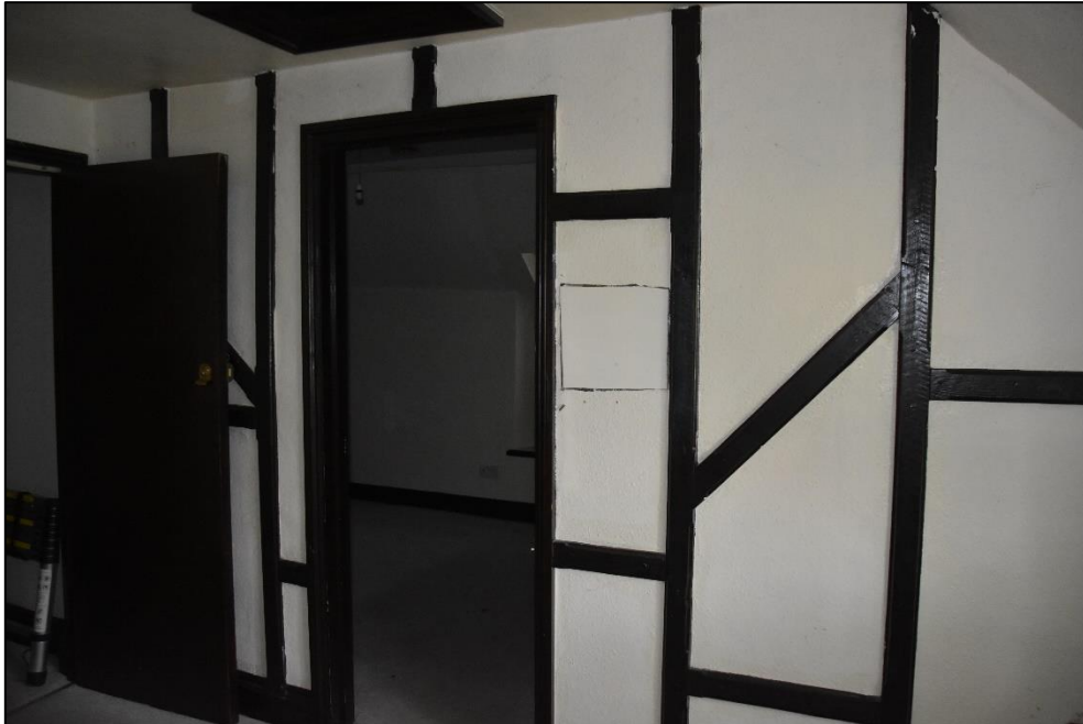
Fictive timber-framing to the south wall of a first floor bedroom (FF05), looking south-west Fig 83
