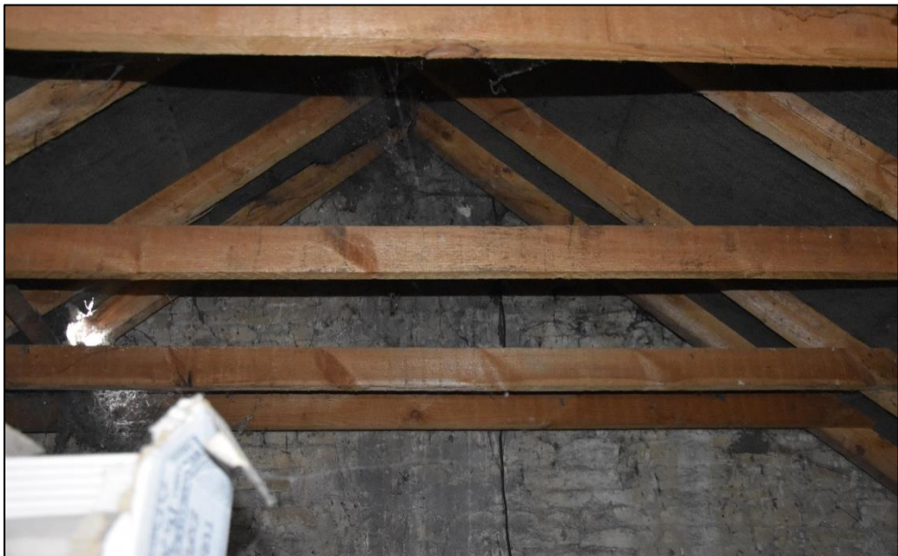
The roof over Range 3, and the west gable end of Range 3, looking west Fig 101
