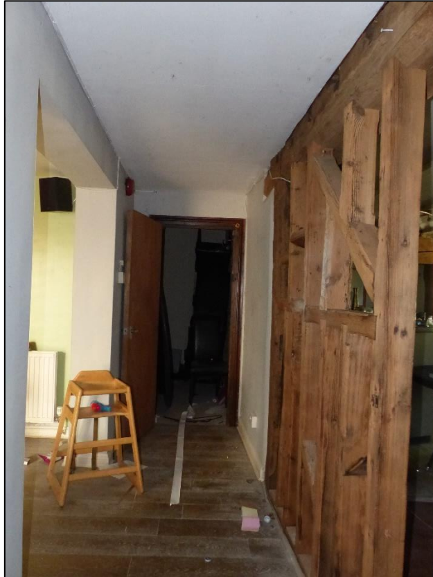
Access corridor (GF05) open to restaurant waiting areas to the east and the lounge to the west, looking north-east Fig 37
