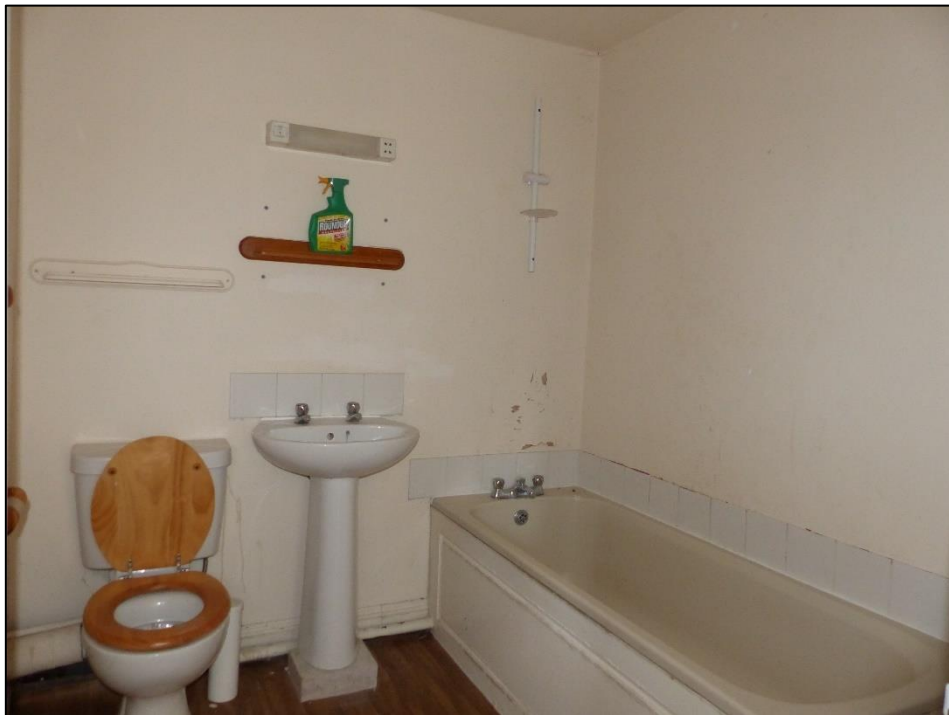
Ensuite to one of the first floor bedrooms (FF07), looking north-east Fig 88
