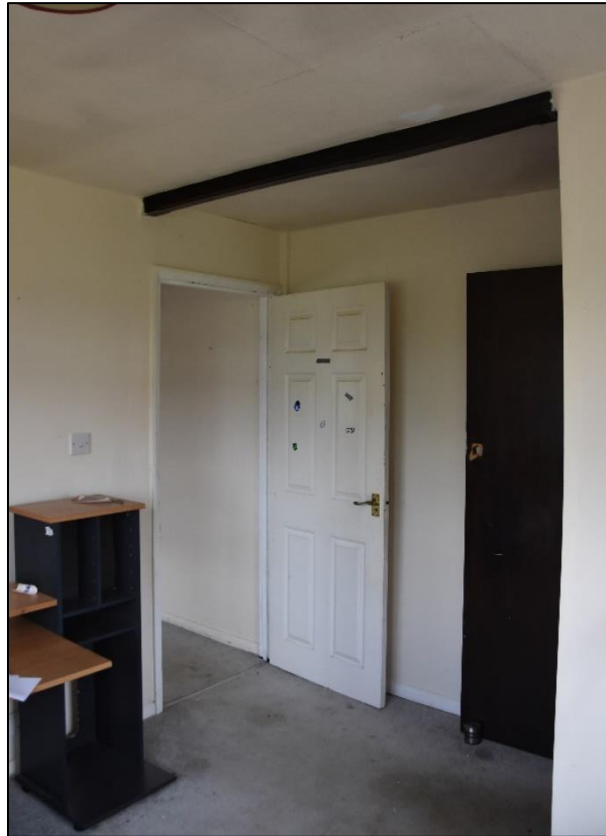
Access from the rear corridor (FF06), and access into the second office (FF10), looking south-east Fig 90
