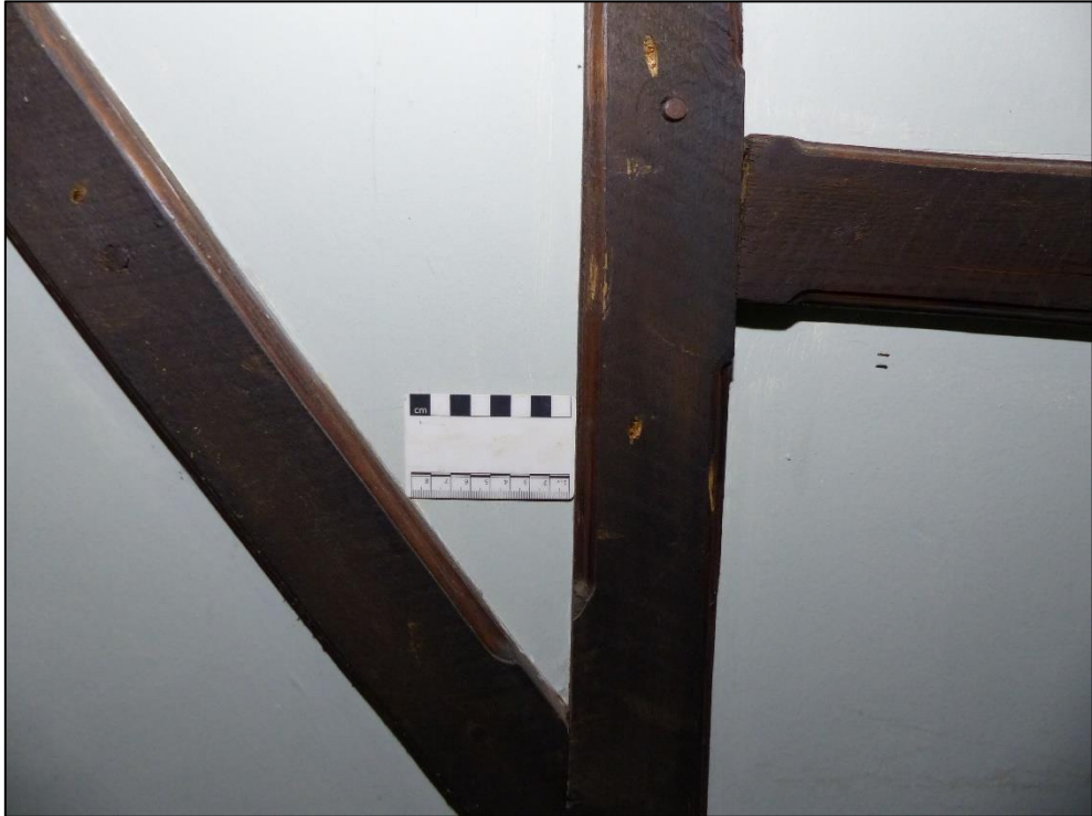
Detail of the fictive timber-framing seen in the lounge (GF02), with moulded chamfers, run-out stops, and pegging, looking north-east Fig 34
