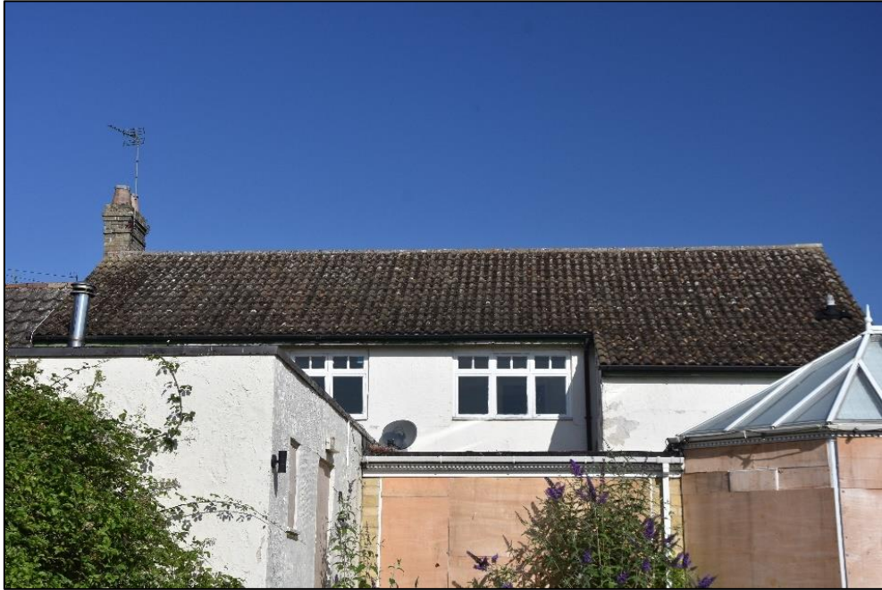
Range 5 to the rear, obscured by Range 6 at ground floor level, looking north-west Fig 15
