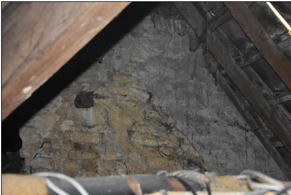
East gable end in the roof over Range 2, showing former roof line of a lower pitched roof, looking south-east Fig 99
