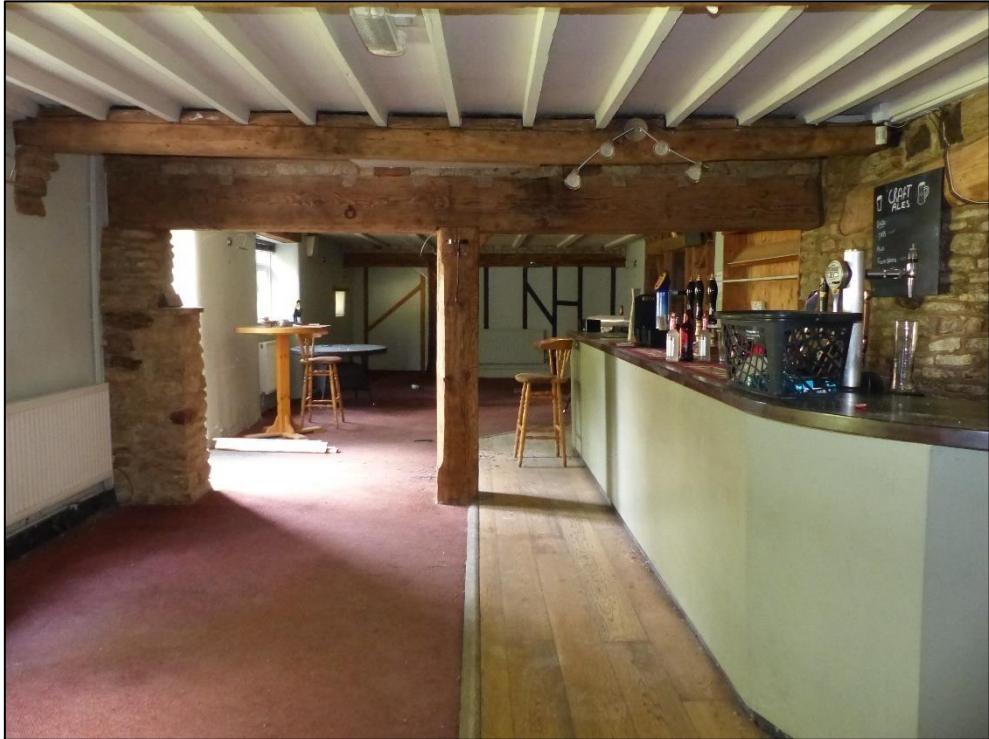
Area to the north of the south bay in the lounge (GF02), looking north-east Fig 29
