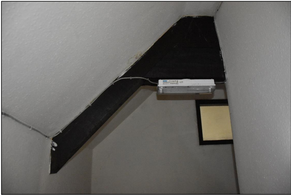
Exposed timber rafter within the first floor corridor (FF01), looking south-east Fig 68
