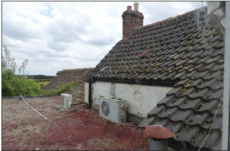
Rear of Range 1 seen from a first floor window, looking south Fig 8
