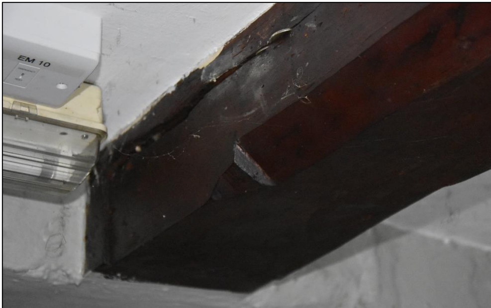
Chamfers and stops to the binding joist in the bar (GF01), looking north-east Fig 25
