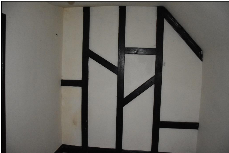
Fictive timber-framing in one of the first floor bedrooms (FF02), looking east Fig 71
