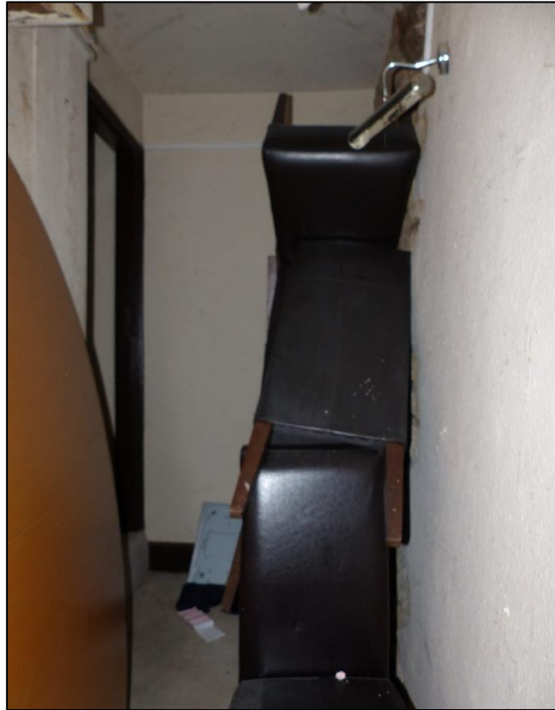
Small stair hall to the south of the main corridor (GF05), looking south-west Fig 38
