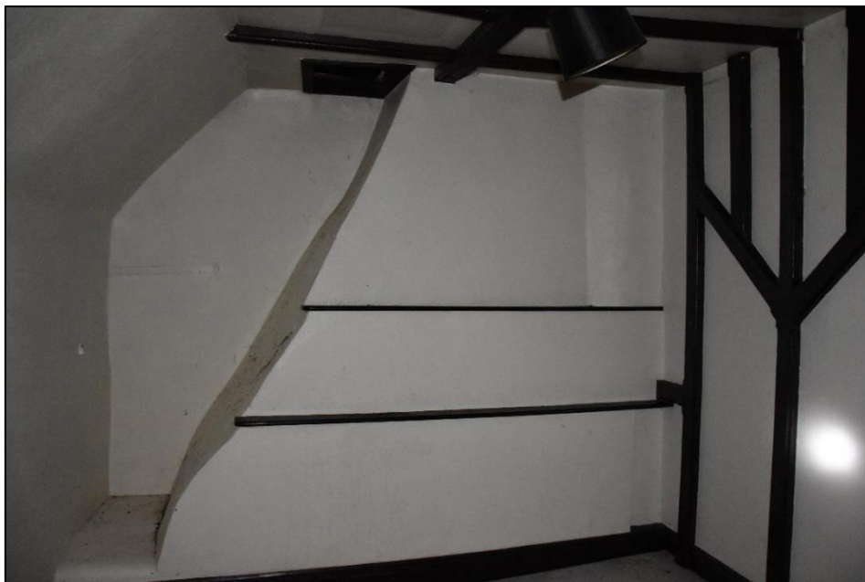
Large stack within one of the first floor bedrooms (FF03), looking north-west Fig 75
