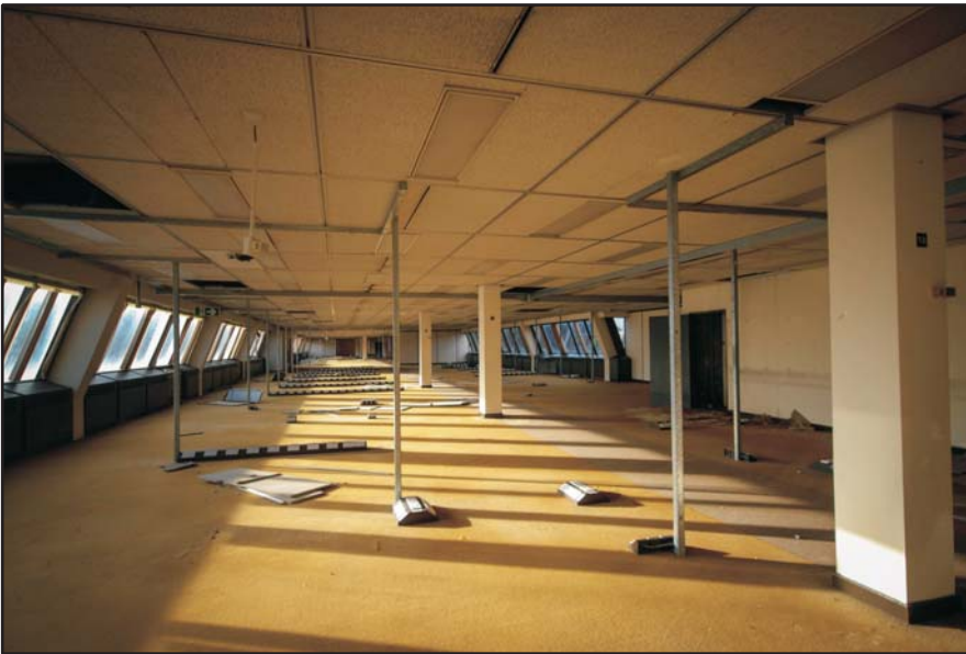
Third Office Level, general view of the office space, looking west Fig 117
