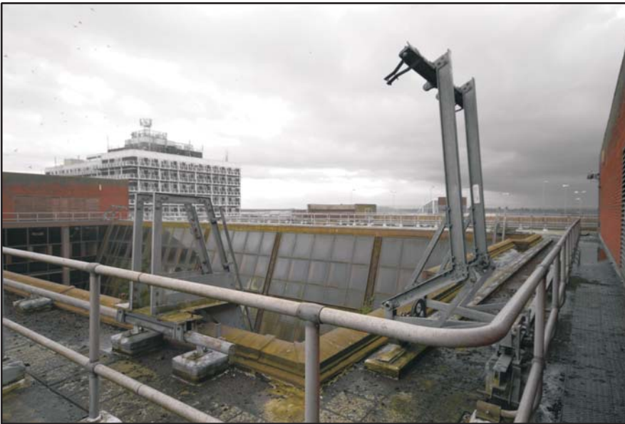
The Roof, East Atrium, detail of the winch, ladder and safety rail Fig 136
