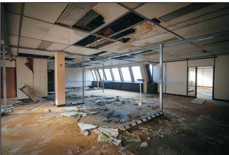
Third Office Level, detail of water damage and mould Fig 119
