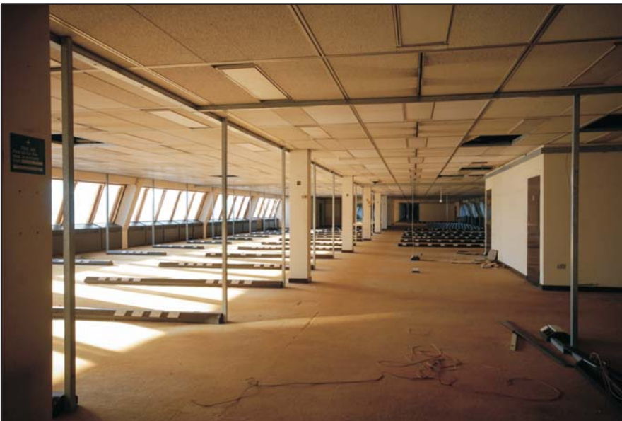
Second Office Level, general view of the office space, looking south-west Fig 110
