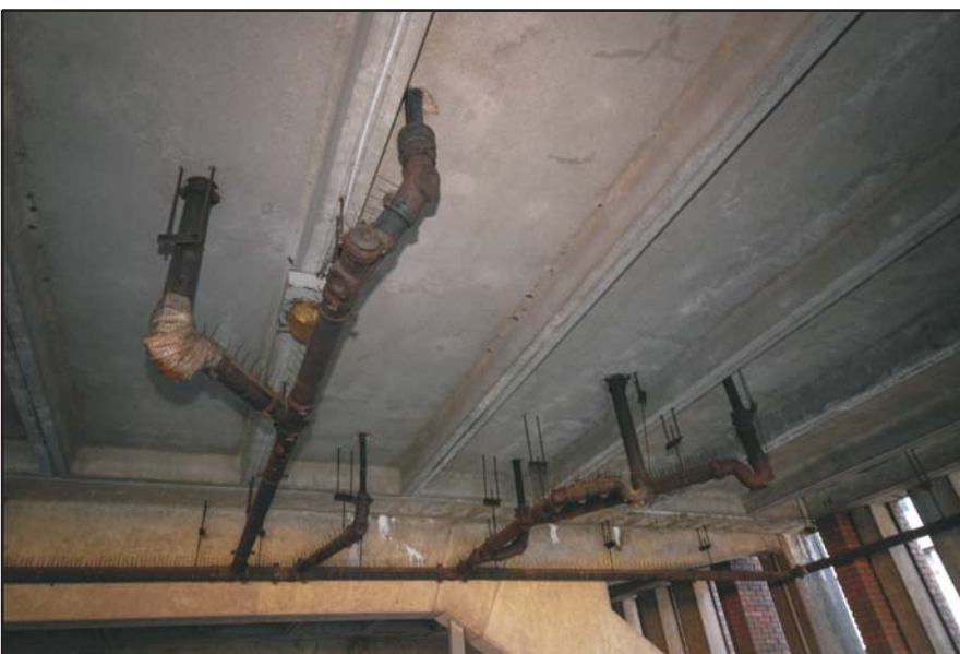
Car Park, detail of pipes on the ceiling Fig 89
