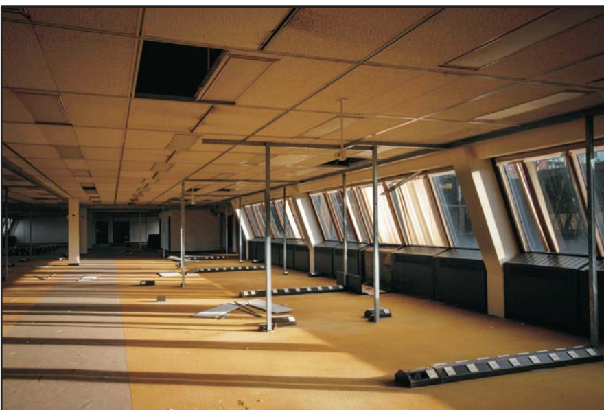
Third Office Level, general view of the office space, looking east Fig 116
