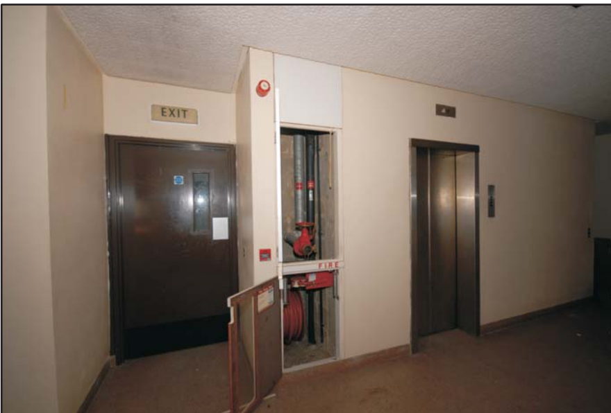
Second Office Level, lift, emergency exit and fire hydrant Fig 106
