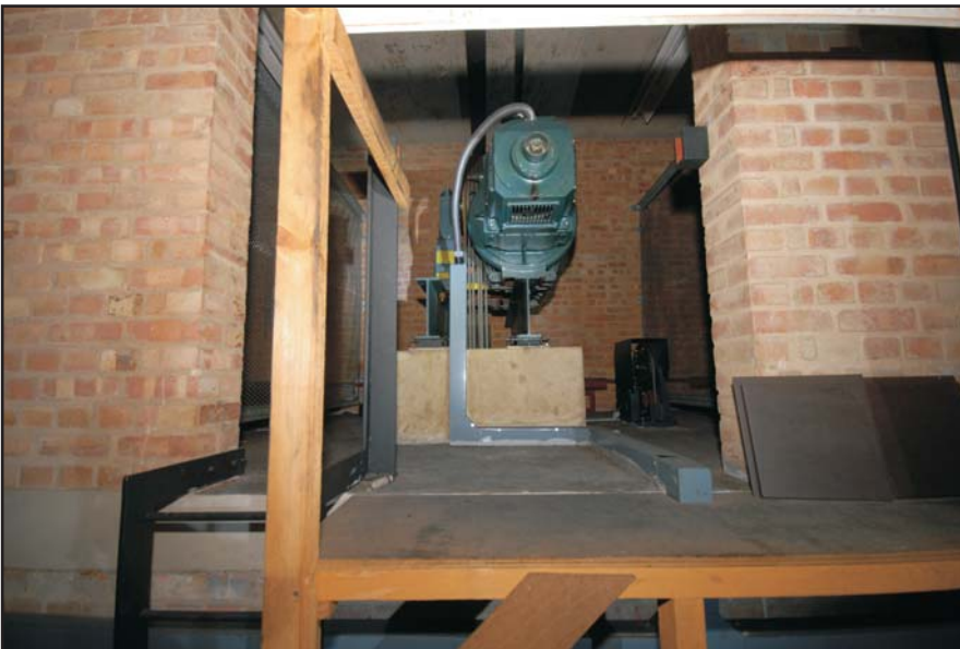
Access Tower, the Plant Room, detail of lift motor Fig 165
