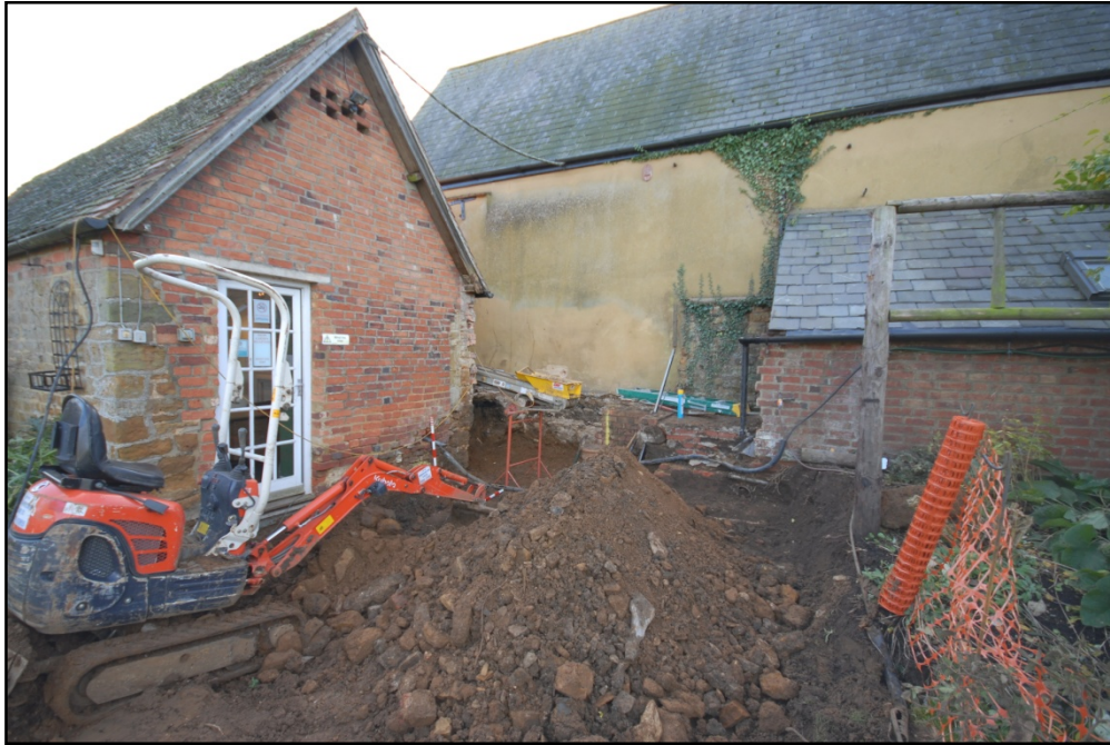
General view of Area 1 at the beginning of groundworks, looking south Fig 7
