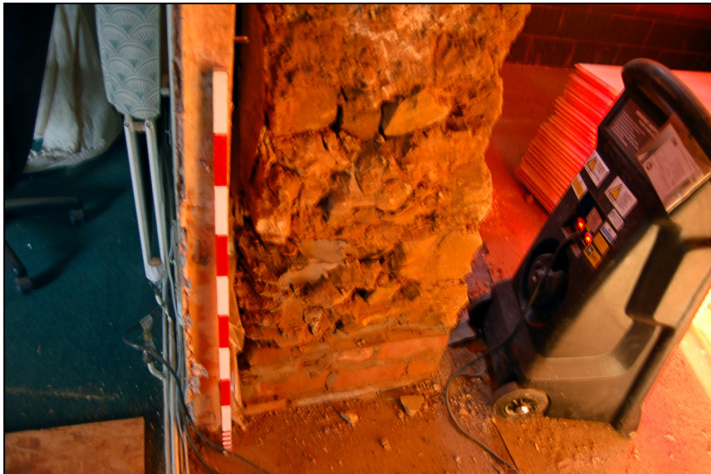
Cross section of the ground floor wall, showing cob with ironstone rubble Fig 20
