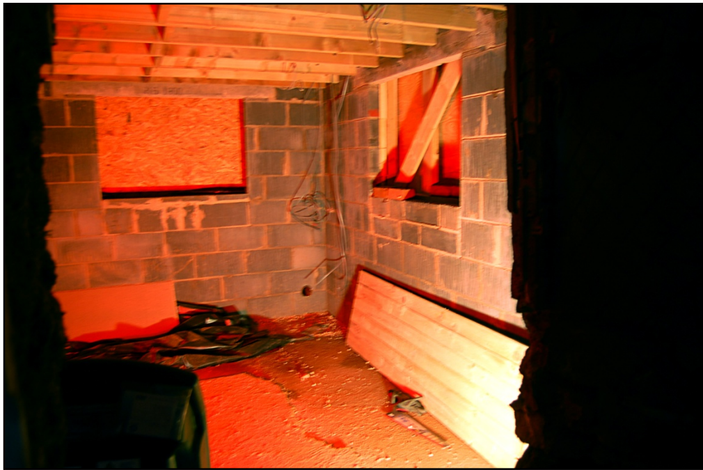
General view of the ground floor of the new extension, looking east Fig 21
