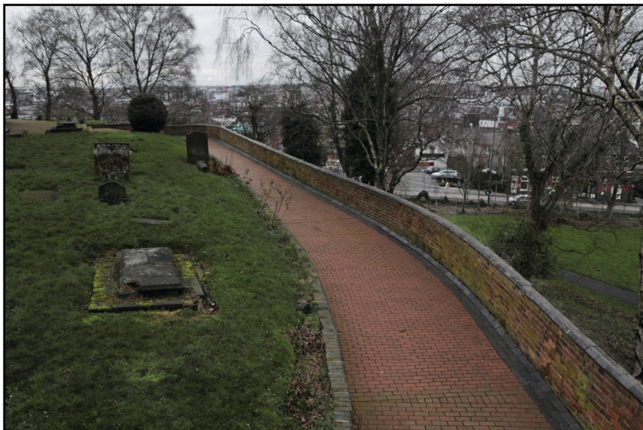
View of the south side of the retaining wall, looking west Fig 20
