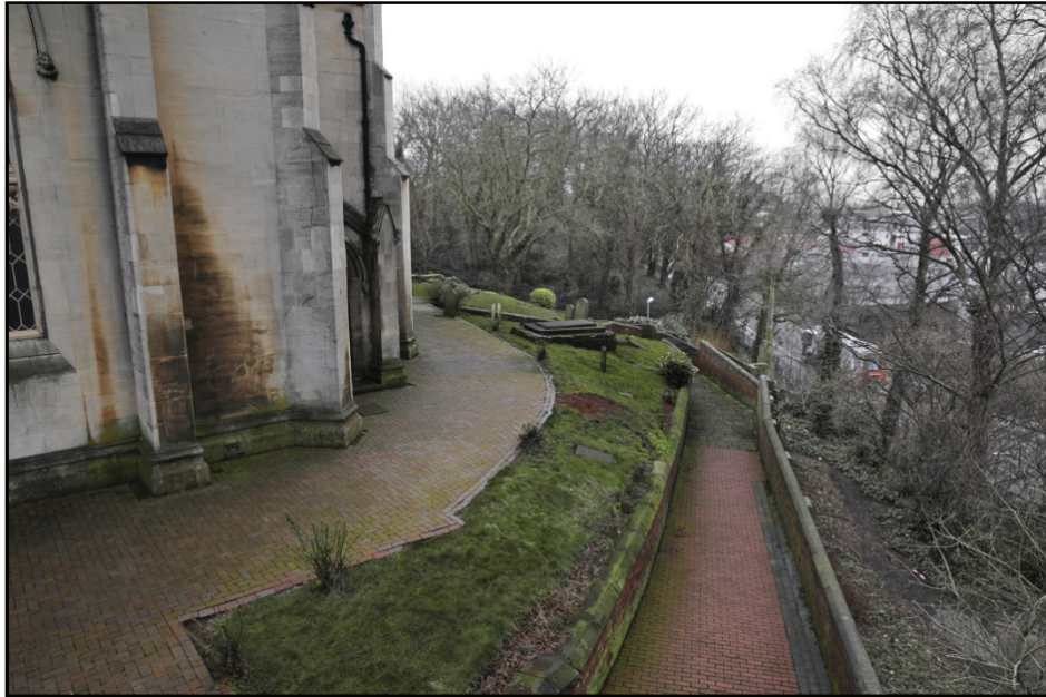
View of the south side of the eastern extent of the retaining wall, looking west Fig 21
