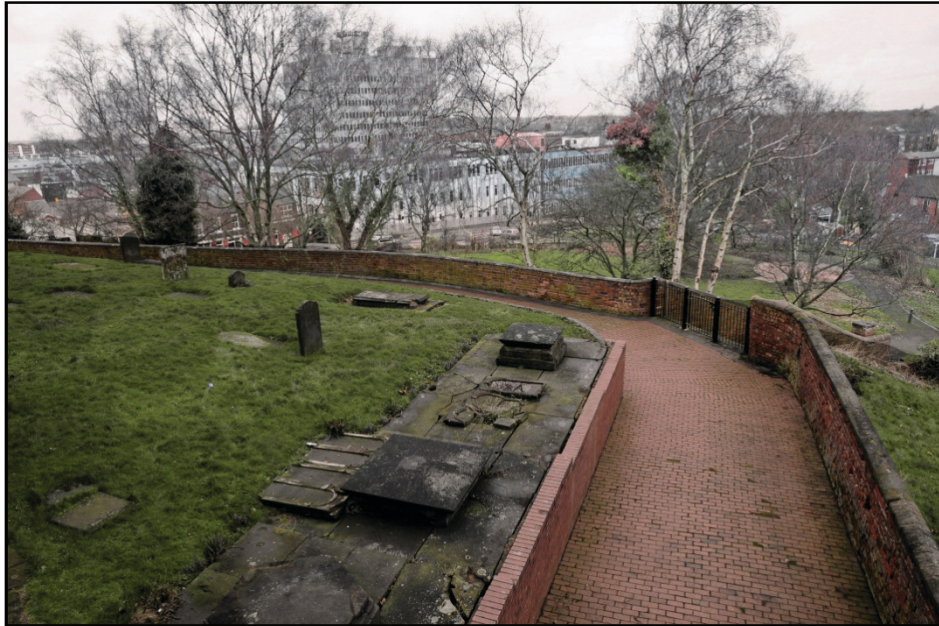
View of the south side of the eastern extent of the retaining wall, looking north-west Fig 19
