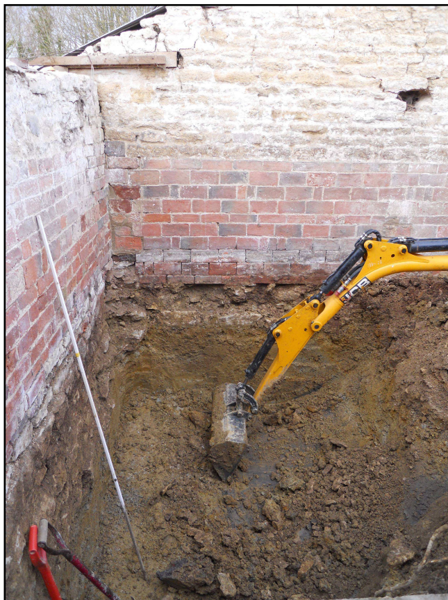
The excavation of the floor in the former garden store, looking east Fig 9
