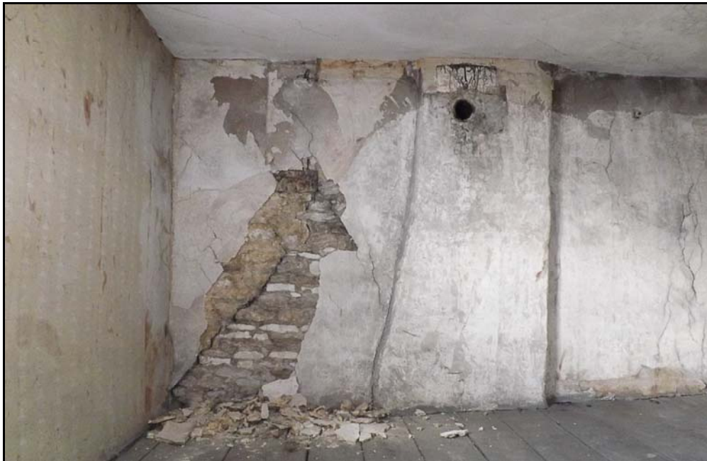
The south elevation with plaster removed, showing the join with original gable Fig 71
